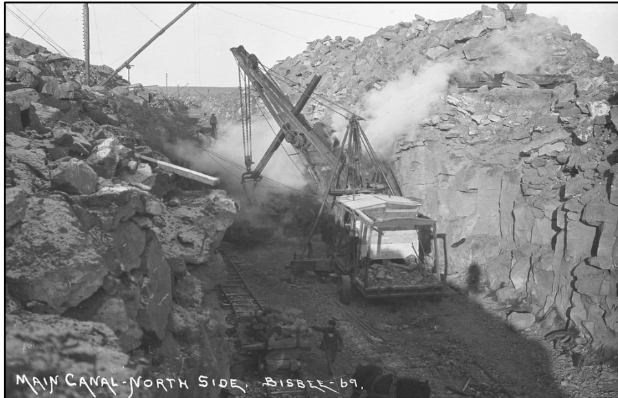
Figure 1-1. A steam shovel digs the North Side Canal from Milner Dam, ca. 1906. Twin Falls Public Library, Clarence E. Bisbee Collection, PC-2084.
