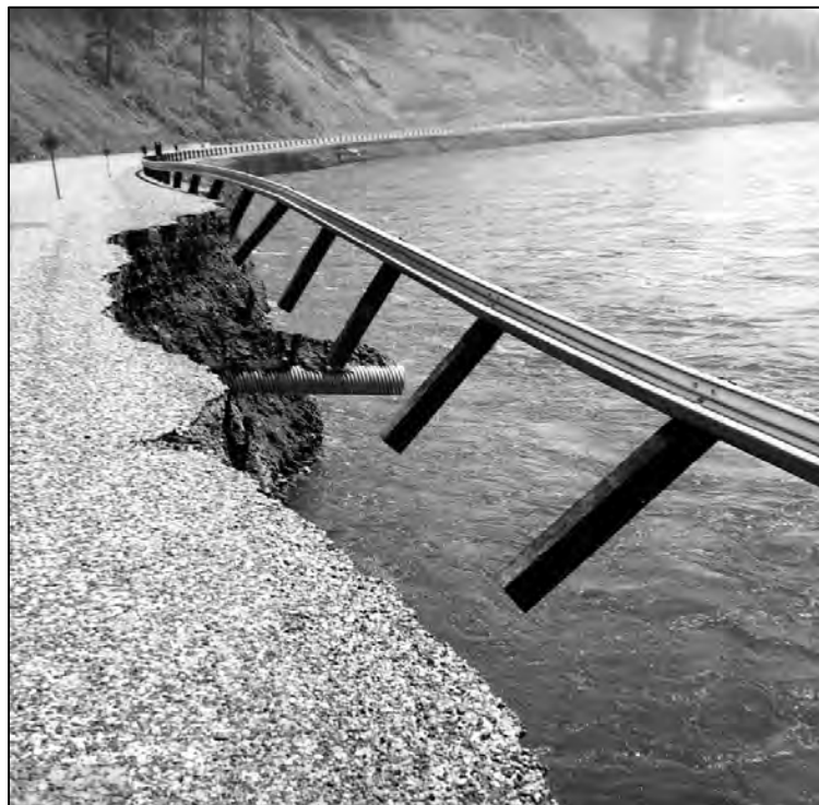
Figure 116. Flooding on US-12 near Kooskia in May 1964 washed out a portion of the highway and guardrail. 573
