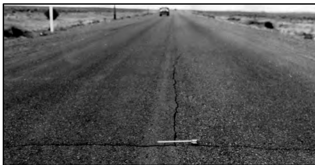
Figure 49. Image from a surface inspection of an access road to Mountain Home Air Force Base, c.1945.. 290
