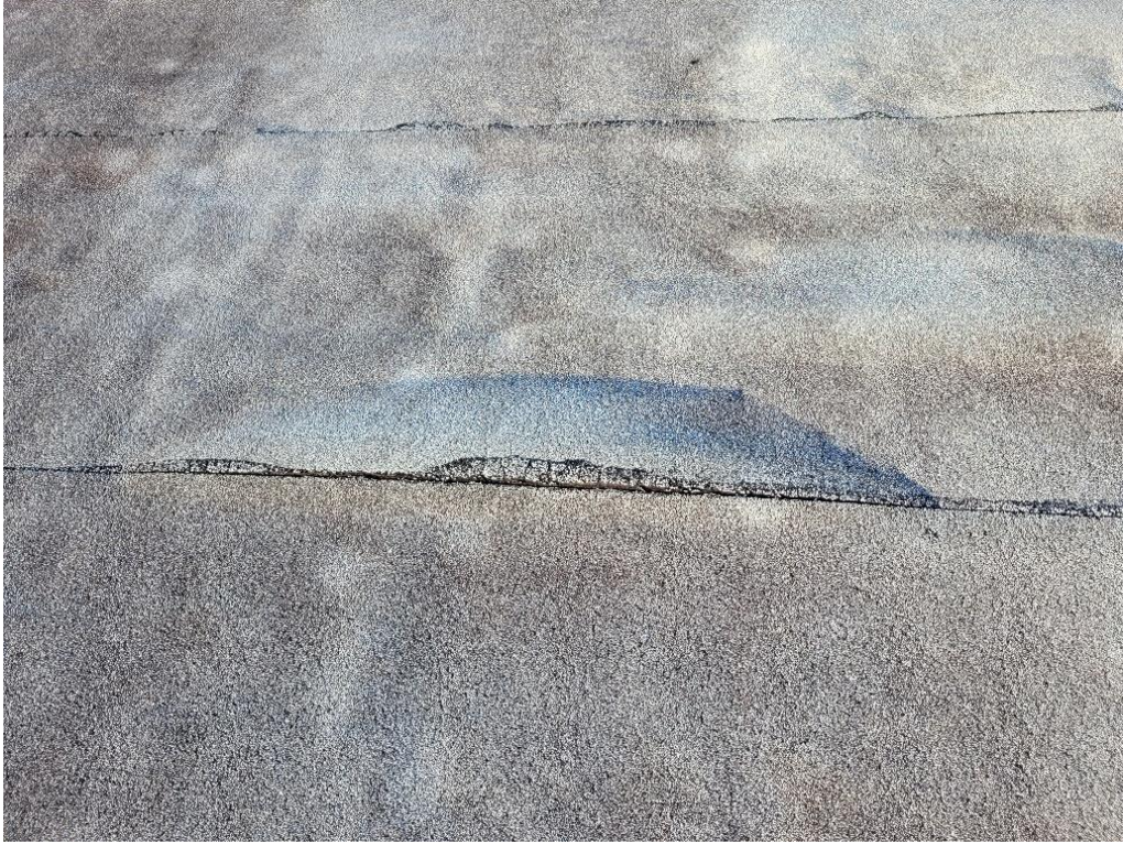
Roof membrane system delaminating and holding water due to the roof exceeding its 20 year design life.
