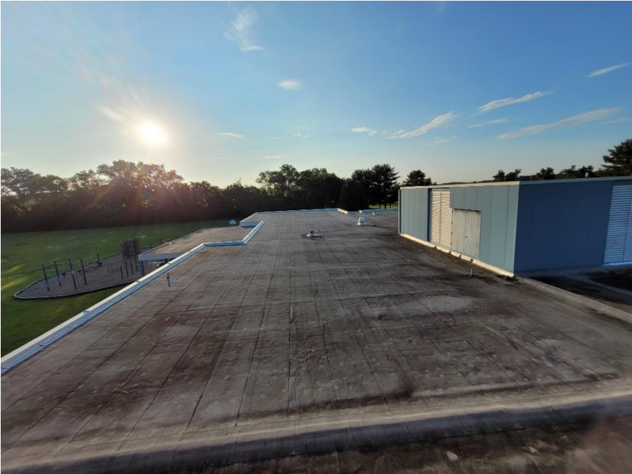
Typical roof facet at WES. Note bitumen bleed out at every seam due to UV protection being lost over 25 years.
