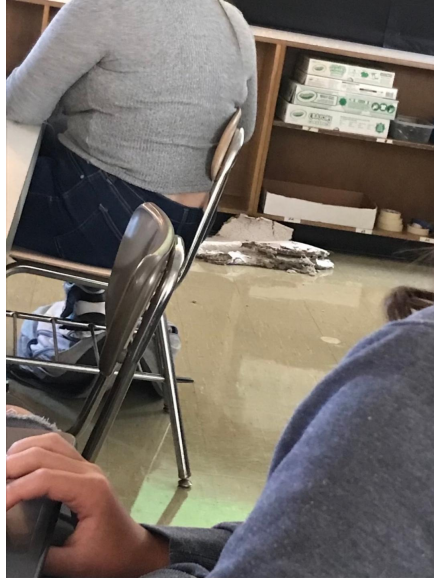
Picture of saturated ceiling tile that fell during instruction.
