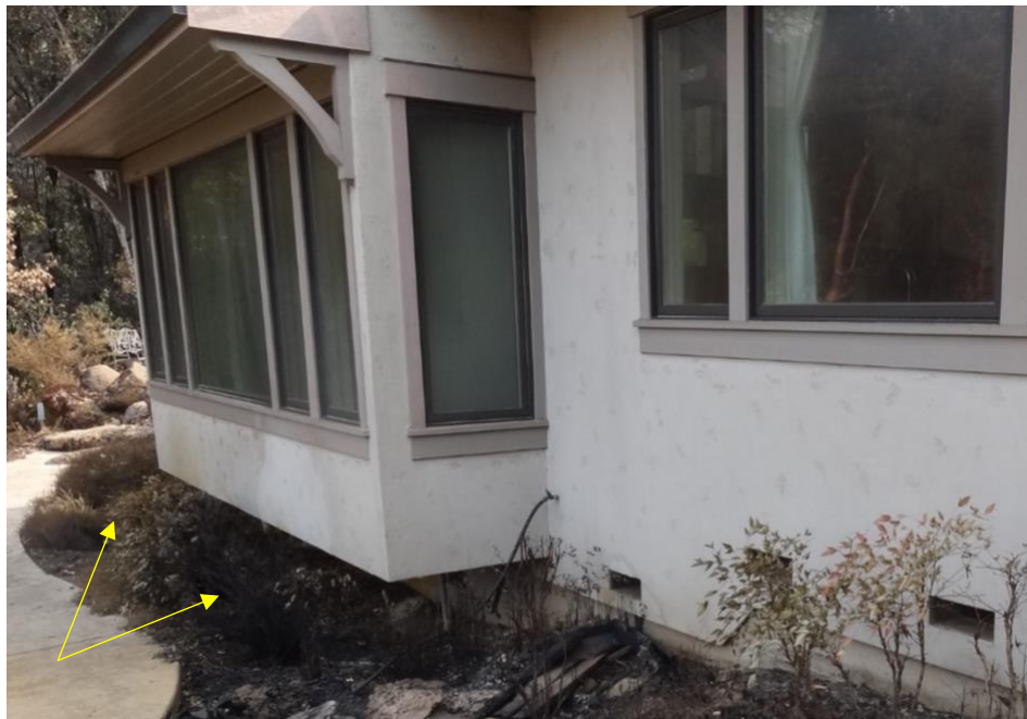
Figure 15. Heat trapped underneath bay windows caused the vegetation in this area to burn disproportionately to its surroundings during the Glass Fire (2020) in Napa and Sonoma Counties, California.
