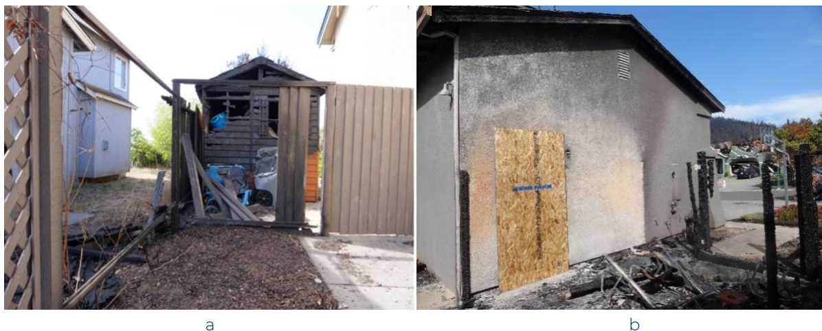
Figure 8. Example of a shed damaging the main structure on a parcel in the Glass Fire (2020) in Napa and Sonoma Counties, California. In photo (a), a shed was about 6 ft away from the main structure (suppressed by first responders and the homeowner). In photo (b), an attached outbuilding completely burned and damaged the main structure (suppressed by first responders).
