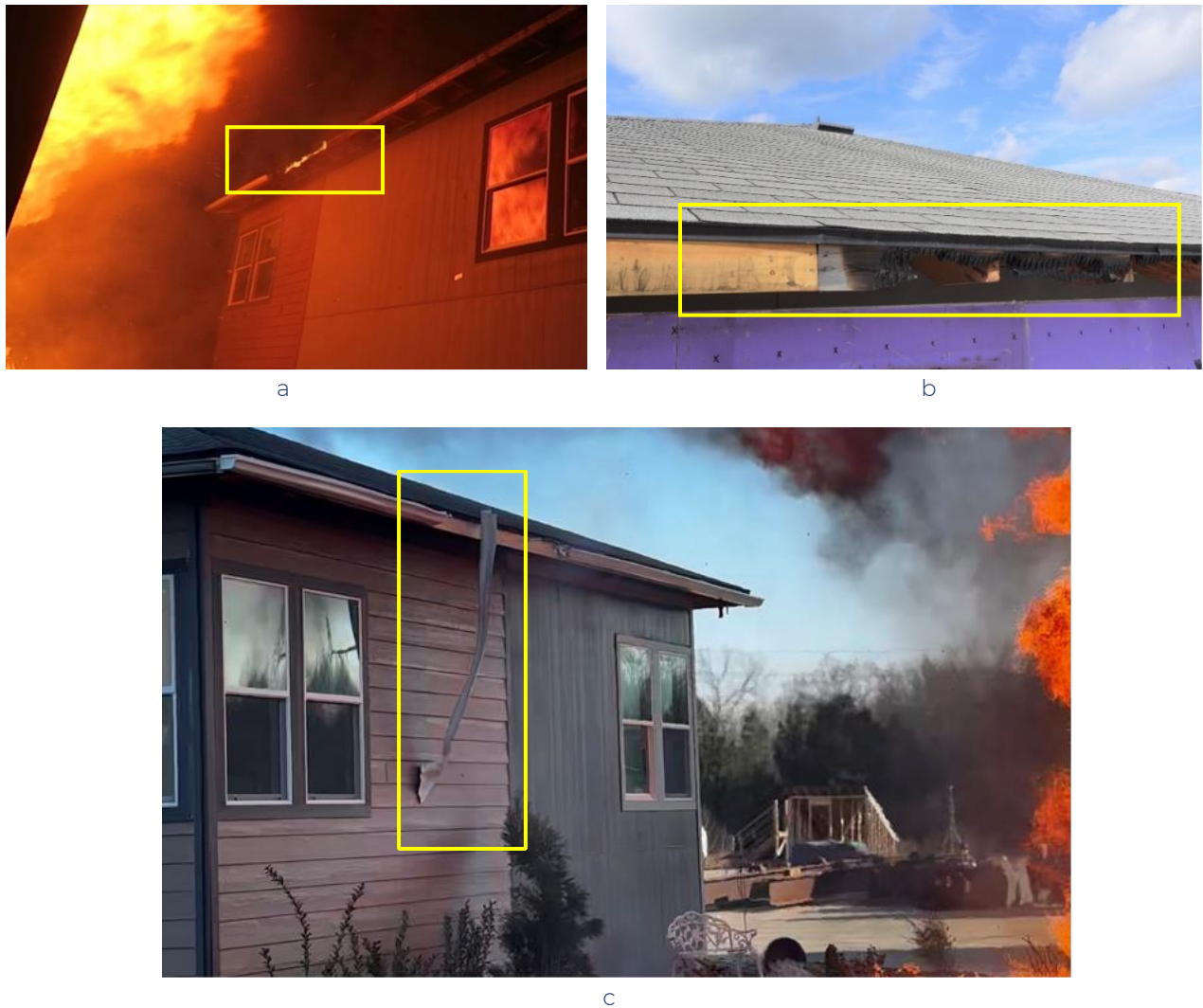
Figure 2. A noncombustible gutter can provide protection for the fascia board if a metal drip edge is not installed. (a) shows fascia board ignition during the experiment and (b) shows the fascia board condition after the test. In (c), a vinyl gutter deformed due to radiant heat/intermittent flame contact and fell off.
