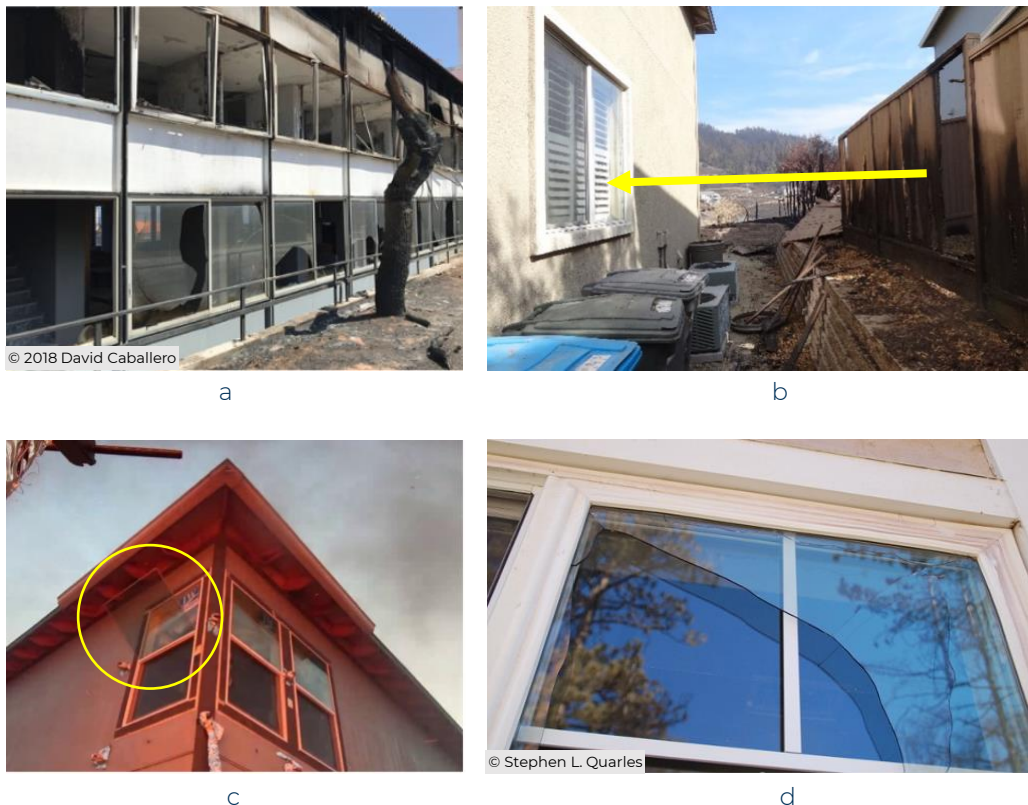
Figure 13. Vulnerability of windows: (a) glazing collapsed in Neos Voutzas-Mati, Greece (2018) due to the combustion of a pine tree (Peñalozza et al., 2021), used with permission; (b) windows damaged by radiation from a burning fence about 10 ft away during the Glass Fire (2020) in Napa and Sonoma Counties, California, where the arrow indicates the direction of radiation; (c) the outer tempered pane of a window fell out during an IBHS full-scale test; (d) window damage following the Grass Valley Fire (2006) in San Bernardino County, California, due to a burning building about 40 ft away, documented by Stephen L. Quarles.
