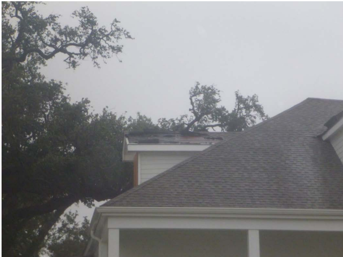
Figure 2.3. Photograph of roof covering loss on a dormer near Bay St. Louis, Mississippi. Photograph by Ian Giammanco, Ph.D.
