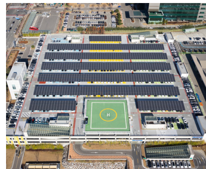
— Installation of solar panels at the rooftops of parking areas in Suwon
