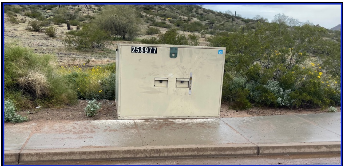
Figure 6 - Ground Mounted Electrical Transformer along North 83 rd Avenue
