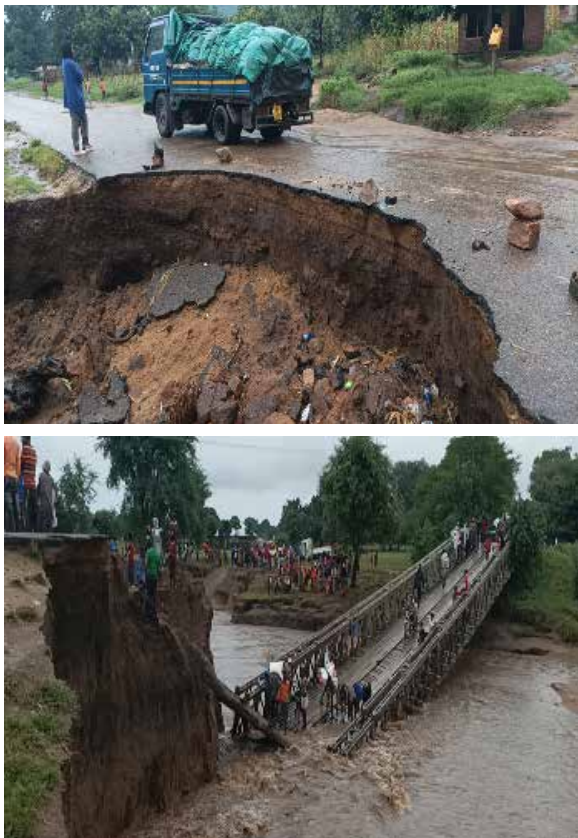
FIGURE 5.9. Image of Road and Bailey Bridge Damaged by Tropical Cyclone Freddy
