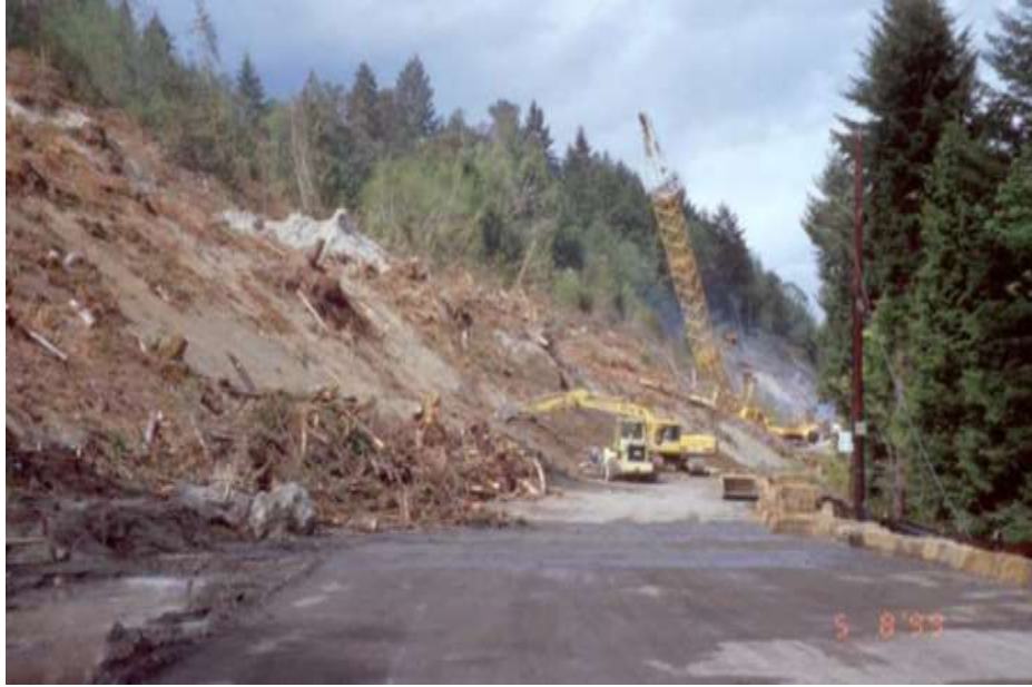
Figure 9-7 Highway Closure at Jorstad Landslide – Winter 1998-1999
