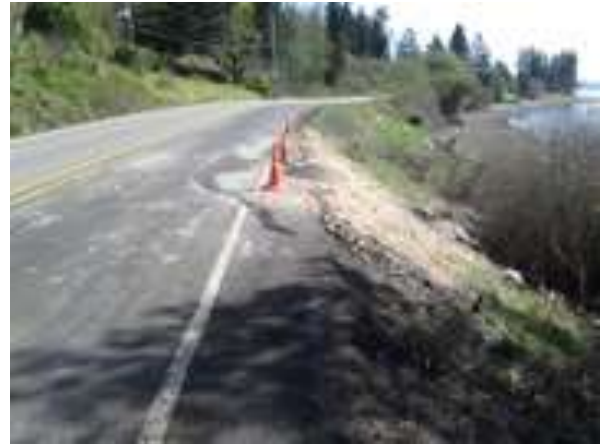
Figure 9-9 SR 302 Slope Erosion
