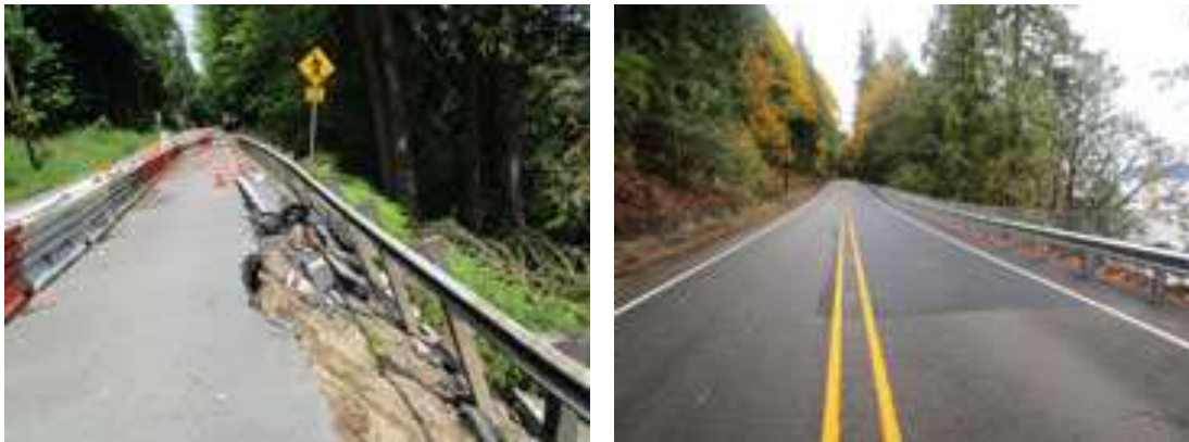
Figure 9-10 Before and After Pictures of SR 101/ 2.2 miles South of Beacon Pt. Road
