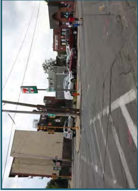
Faded pavement markings at Broadway/Tremont Street intersection
