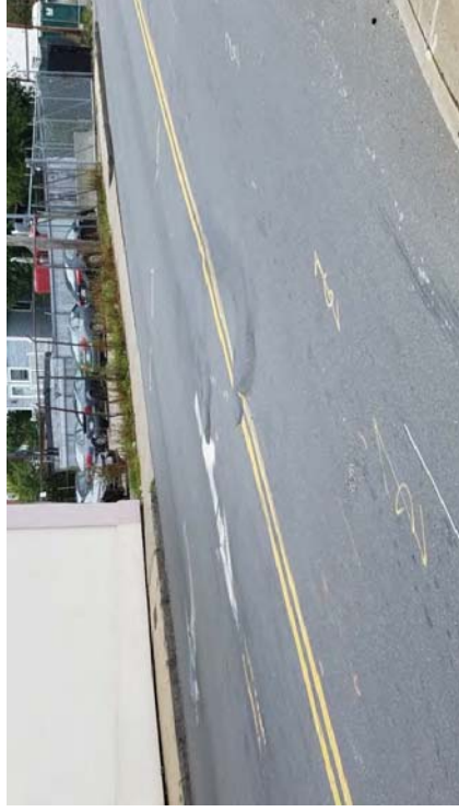
Image 2: Williams Street at Pearl Street – Williams Street approach showing worn pavement markings and rutted pavement.
