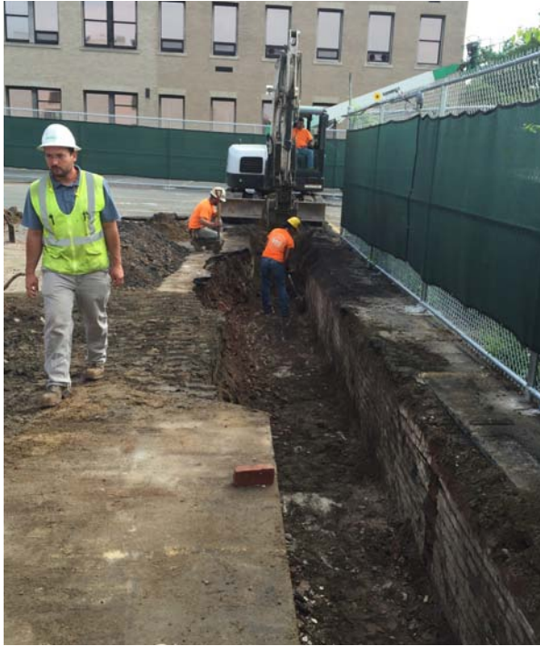
07-15-15 Verizon Duct Bank
