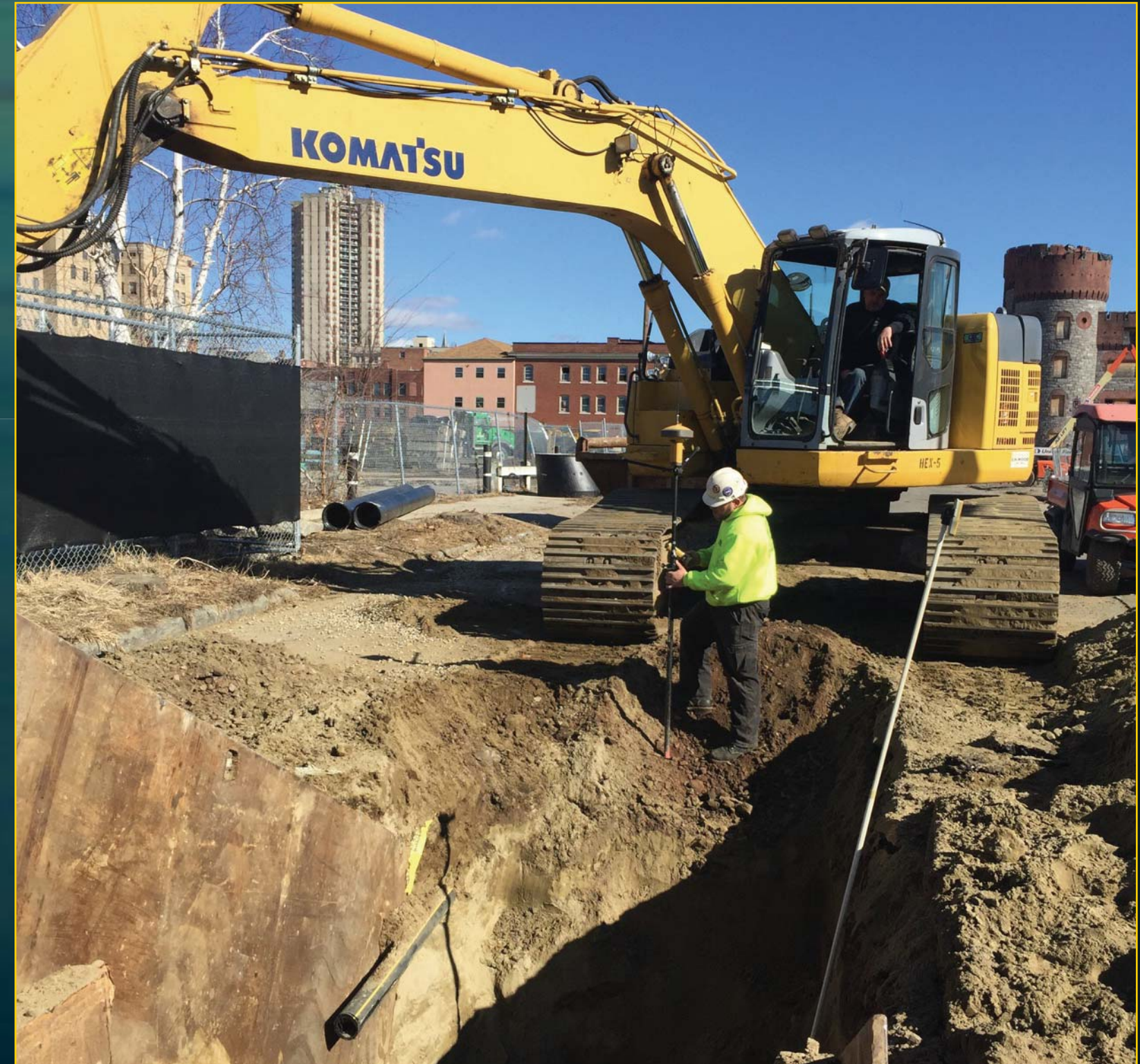
Howard Street Sewer - February 22, 2016
