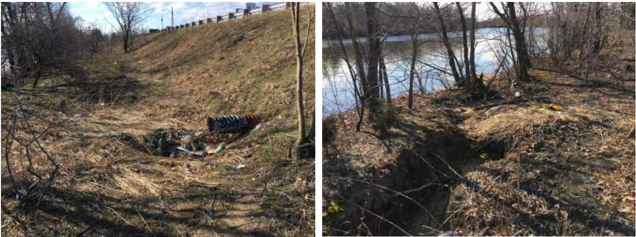
Figures 20 and 21 Existing Stormwater outfalls and observed erosion.
