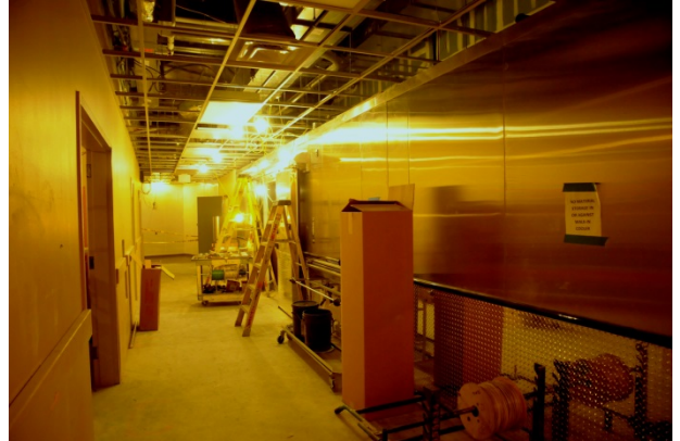
Walk In Coolers Service Area Behind Stage
