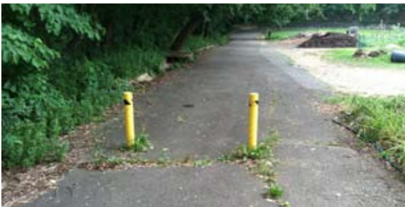
The road behind the community garden is in poor condition. It also has a dead end which causes drivers to conduct a three point turn, often damaging the adjacent wooded area.
