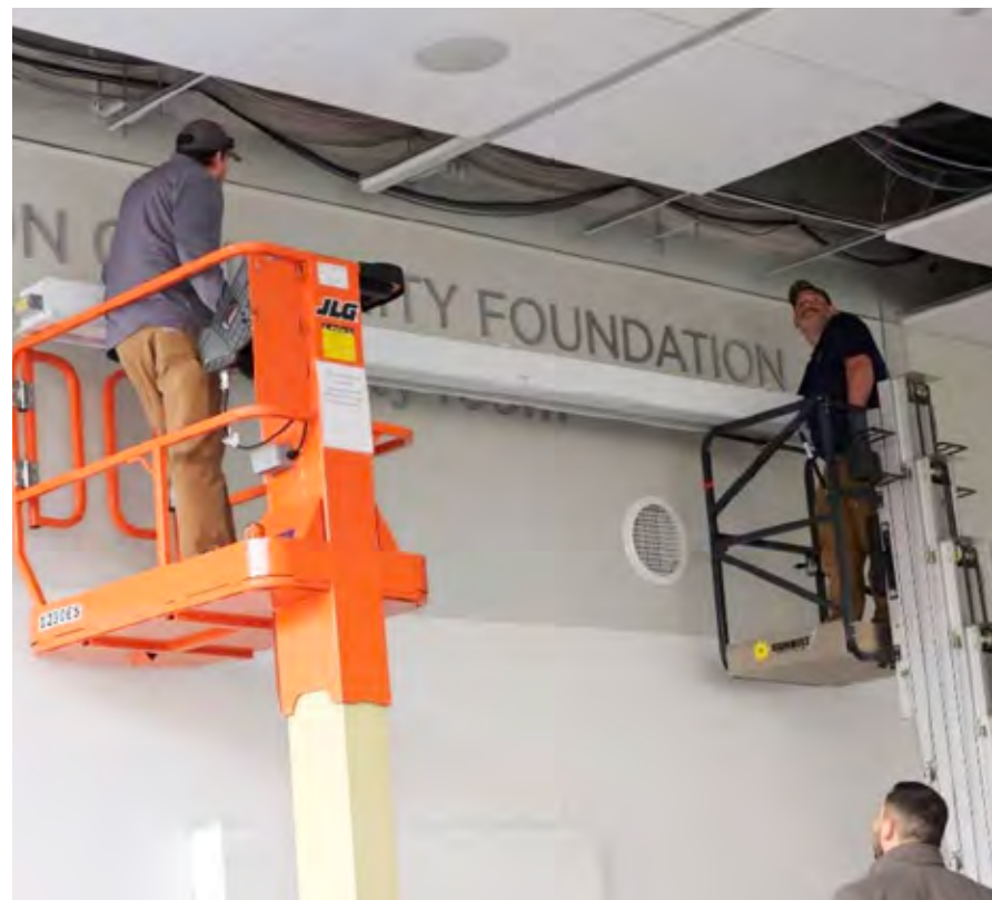
AV equipment installation and wiring in the Community Room at Central Library
