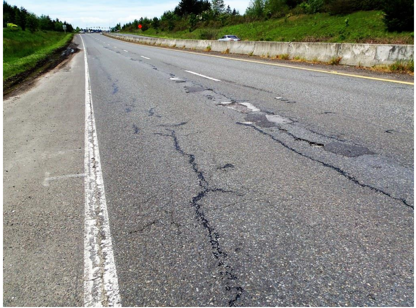
Figure 11. Pavement rutting in Washington State [39]
