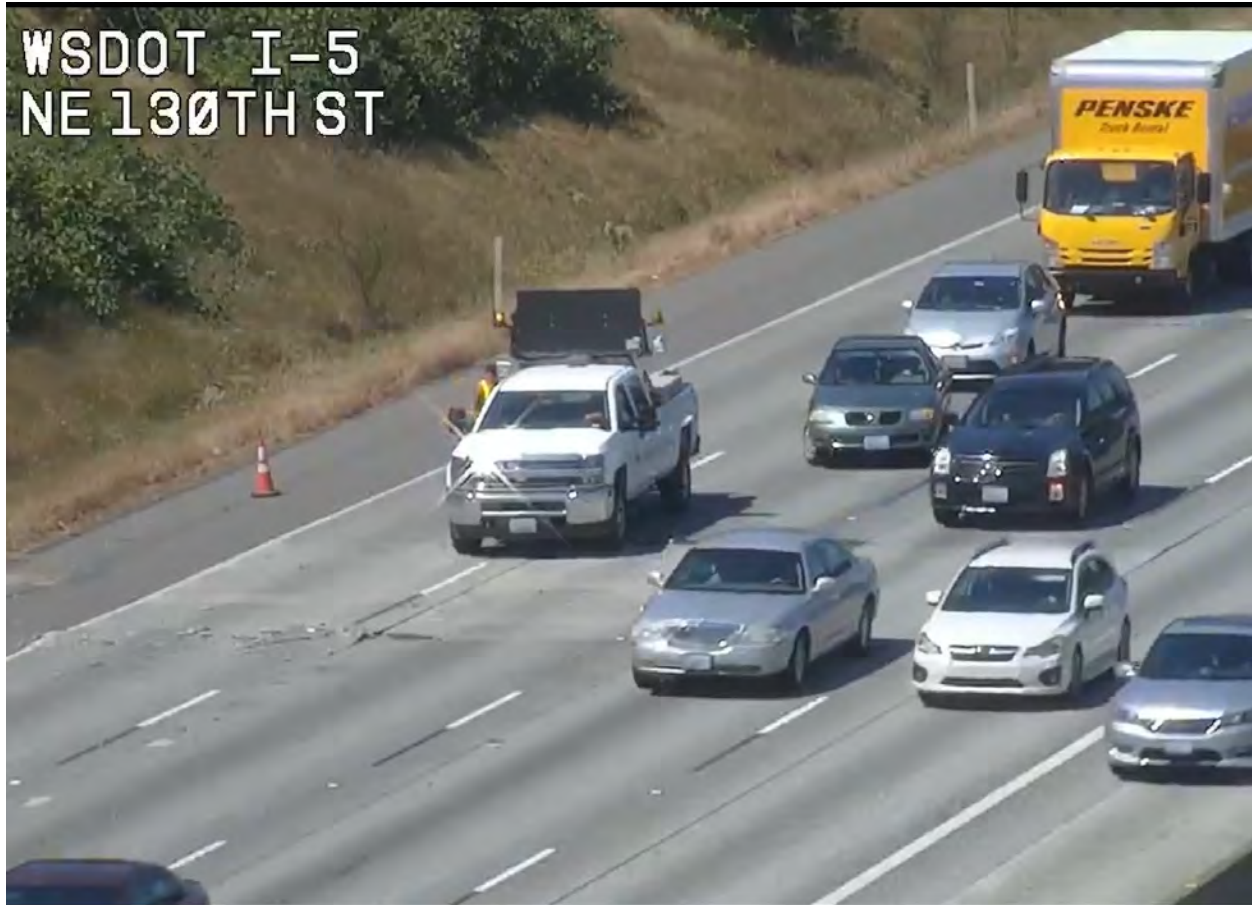
Figure 47. Pavement Buckling During the 2021 Heat Dome Event on Southbound I-5 at NE 130th St.
