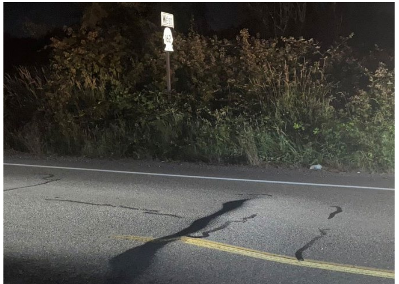
Between June 26-28, 2021, temperatures reached 107°F in South Prairie causing the pavement along SR 162 to warp and elevate nearly four inches. Source: WSDOT
