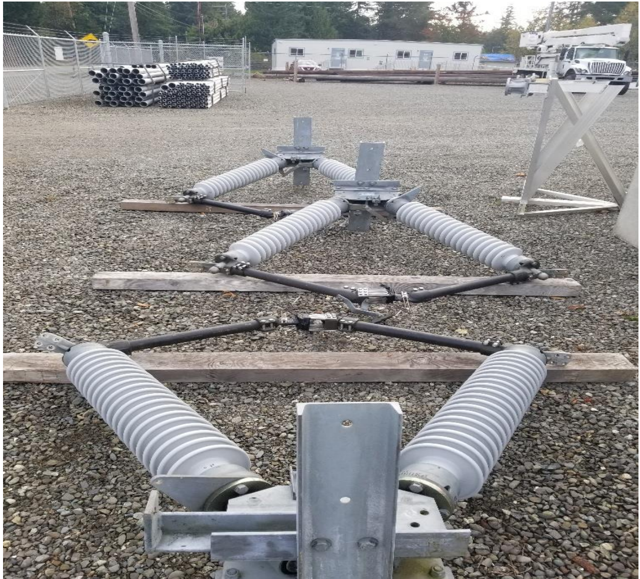
115kV switches old and burned up. Located at 210 Four Corners Road storage yard.
