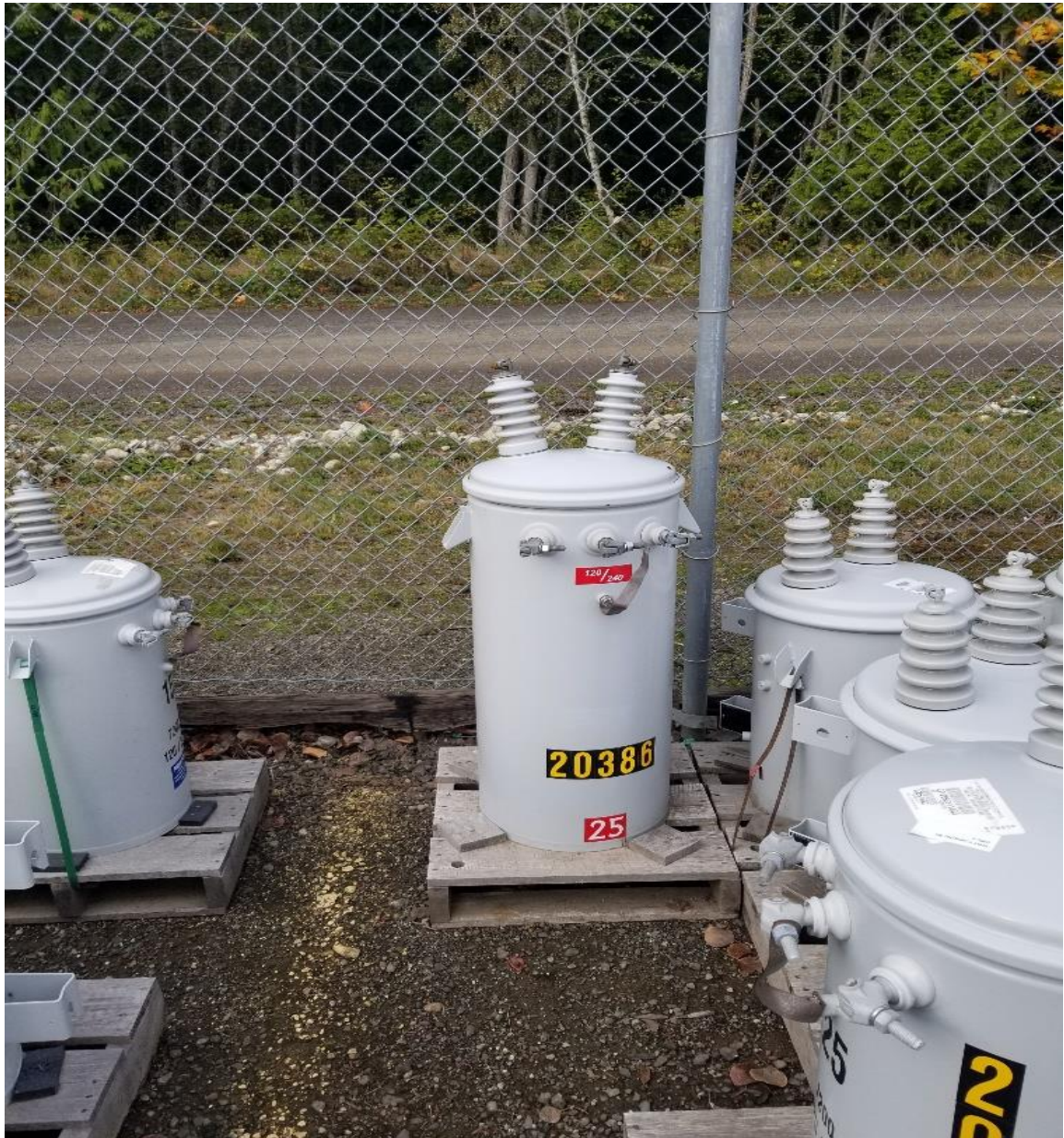
25kV 120/240 transformer west end of Operations center yard.
