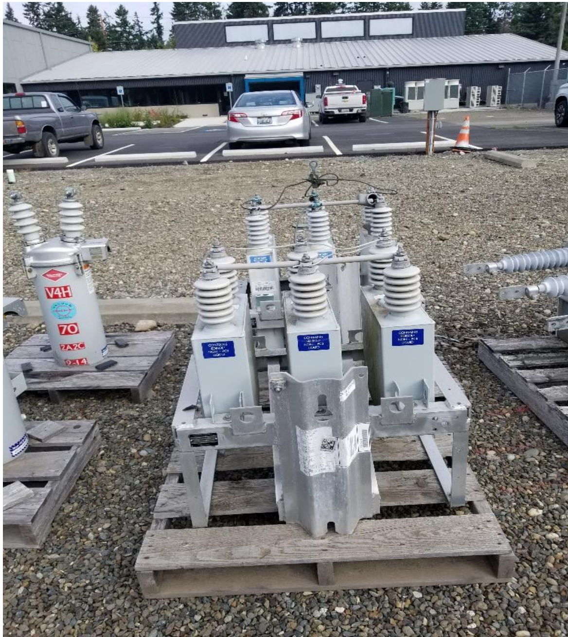
(2) Capacitor banks located near septic system in Operation Center yard.
