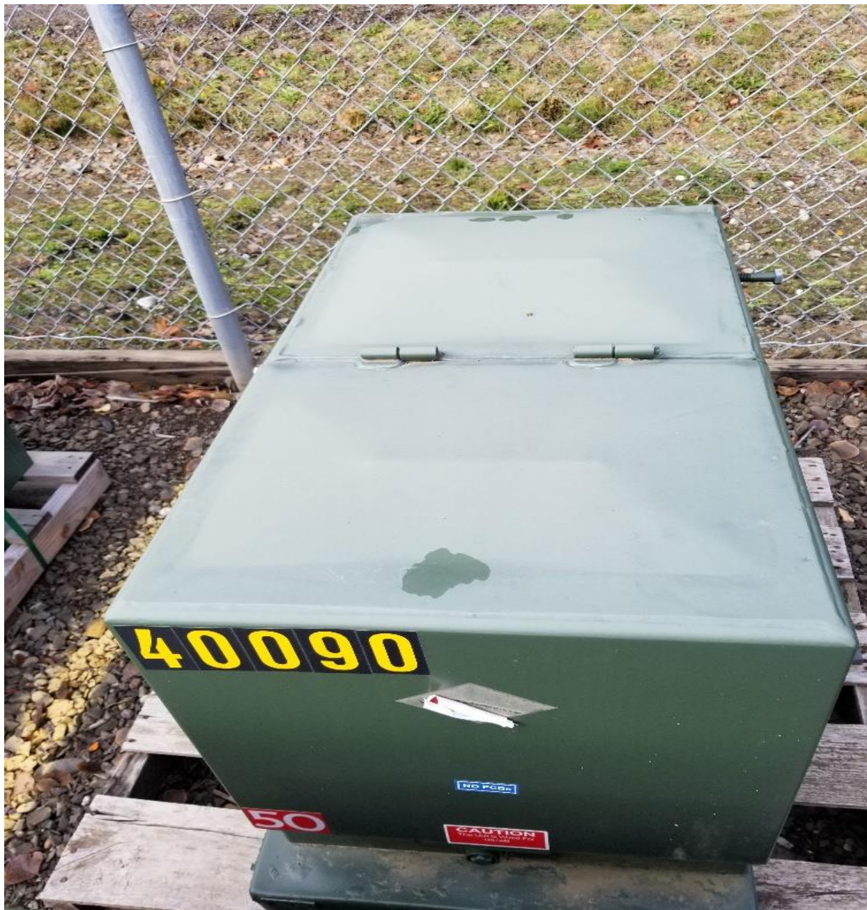
(1) 120/240 50kV transformer west fence line Operation Center yard.
