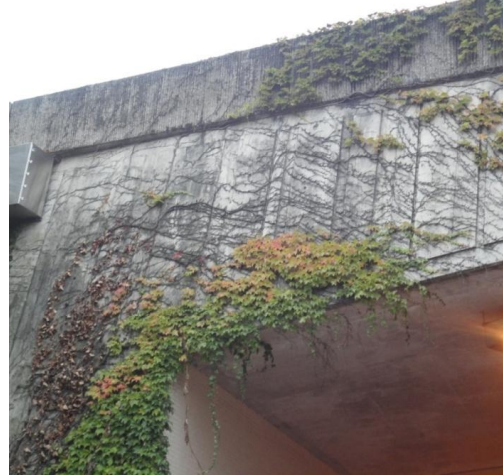
Vines on the walls make a more attractive surface both with and without leaves, adding interest throughout the seasons.
