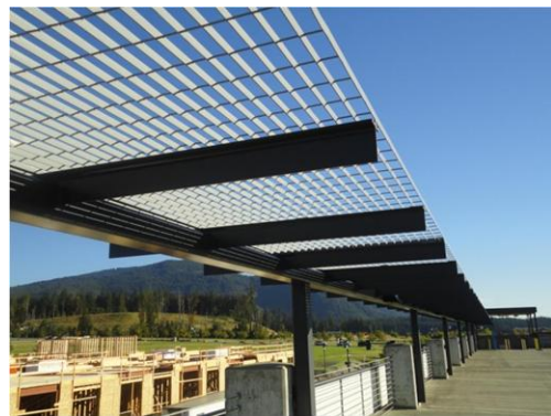
Garage rooftops that are used for parking need to be treated as surface parking lots but the elements do not have to include landscape. Architectural elements can substitute and add to the building's character.
