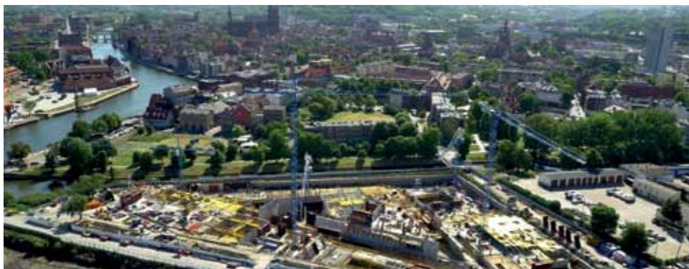
Bird's-eye view of the construction site of the Museum of the Second World War. June 2015. Photo: AeroLab
