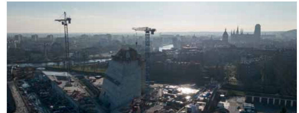
Bird's-eye view of the construction site of the Museum of the Second World War. November 2015. Photo: AeroLab
