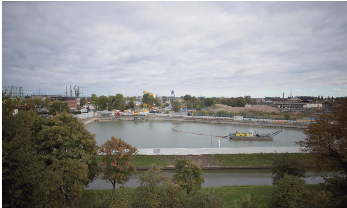
Construction site of the Museum of the Second World War. 7 October 2013. Photo: Roman Jocher
