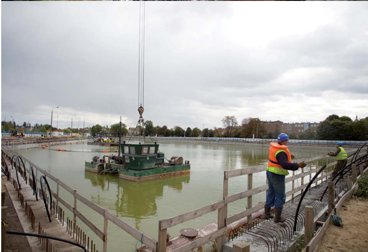
Construction site of the Museum of the Second World War. 27 September 2013. Photo: Roman Jocher
