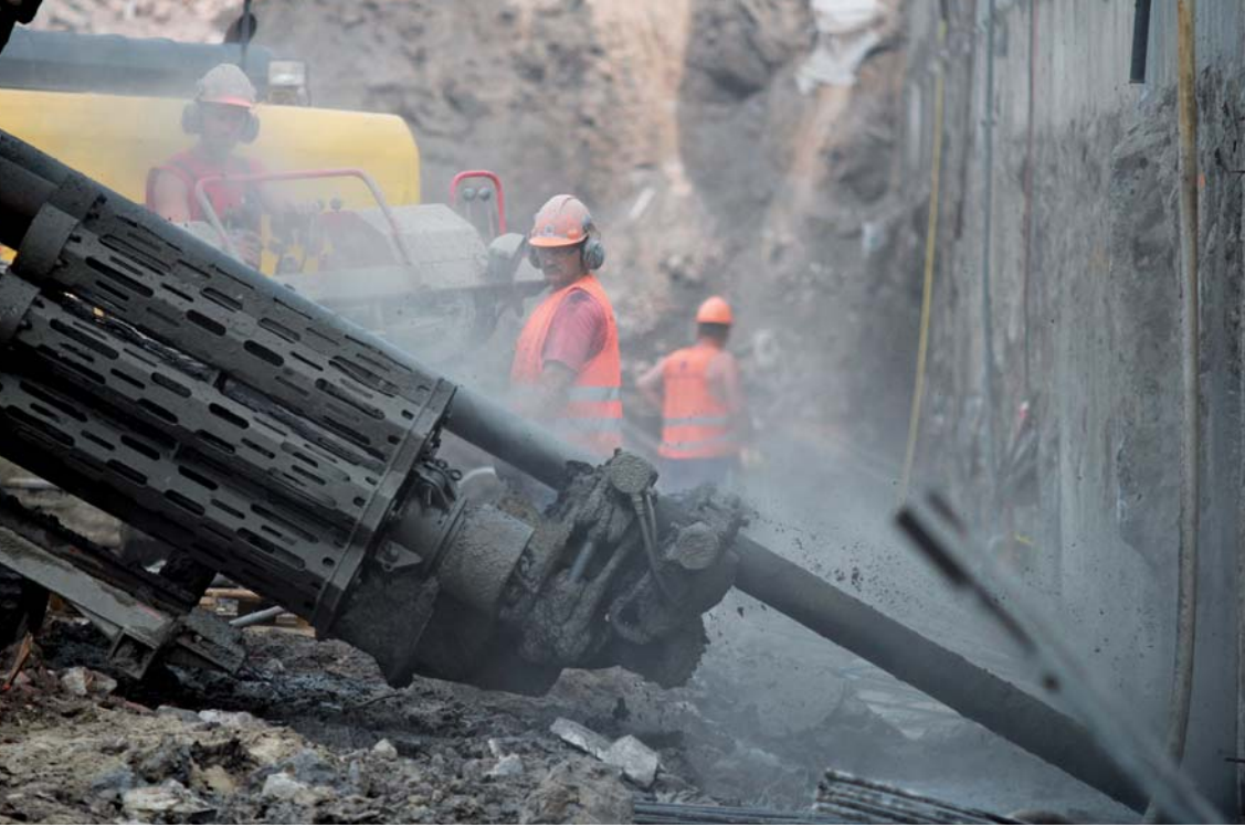
Construction site of the Museum of the Second World War. 8 August 2013. Photo: Roman Jocher
