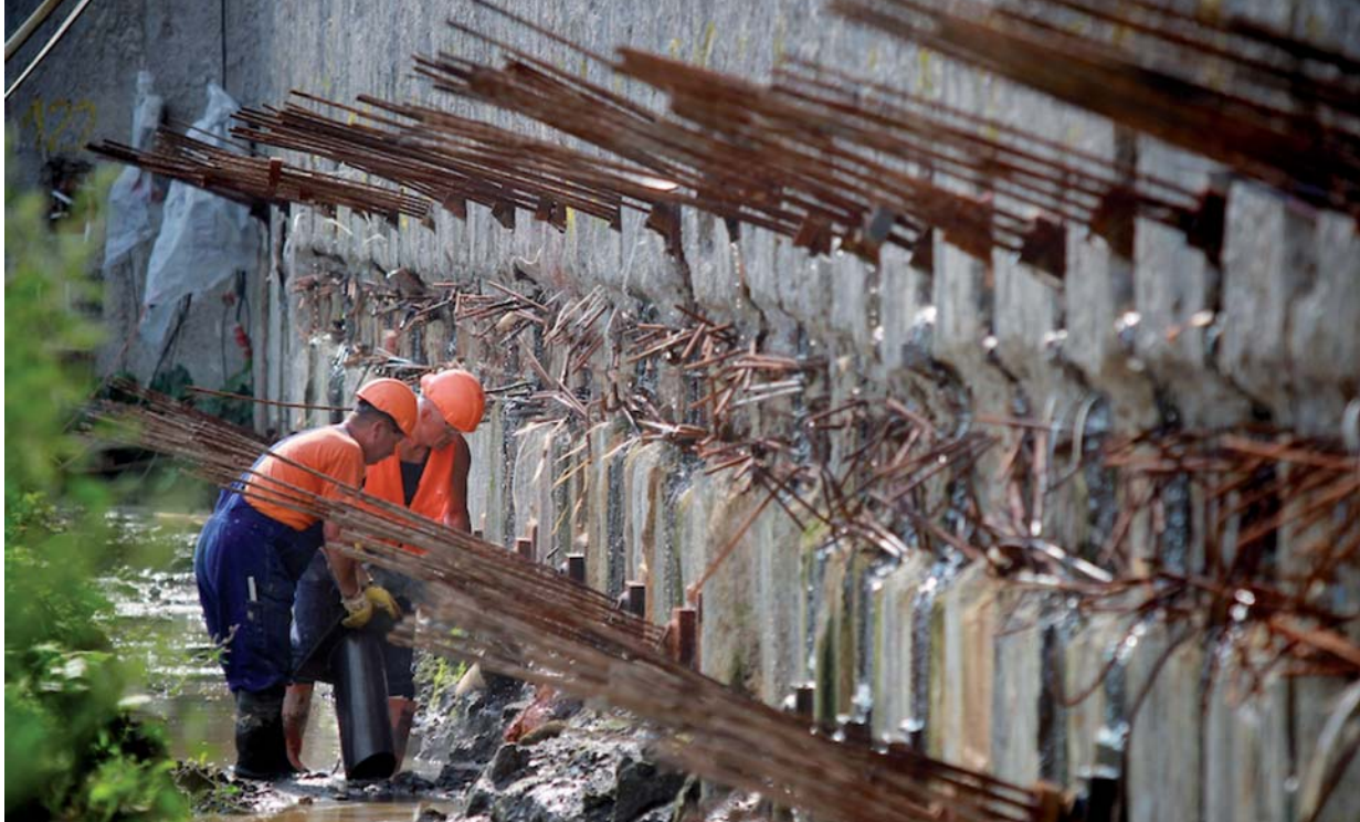
Construction site of the Museum of the Second World War. 8 August 2013. Photo: Roman Jocher
