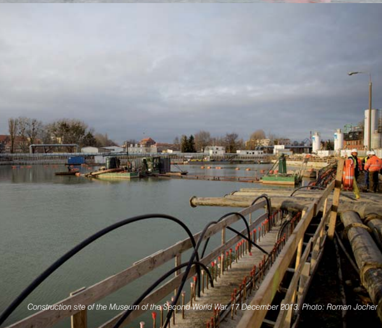
Construction site of the Museum of the Second World War. 7 October 2013. Photo: Roman Jocher
