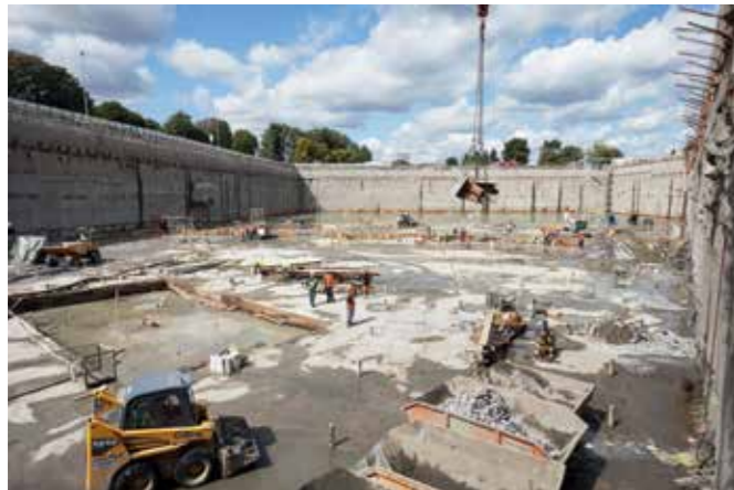
Cleaning and levelling the pit bottom after the water was pumped out
