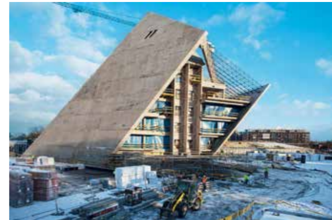
Construction of the Museum tower is finished — preparing the installation of a glass skylight and the façade
