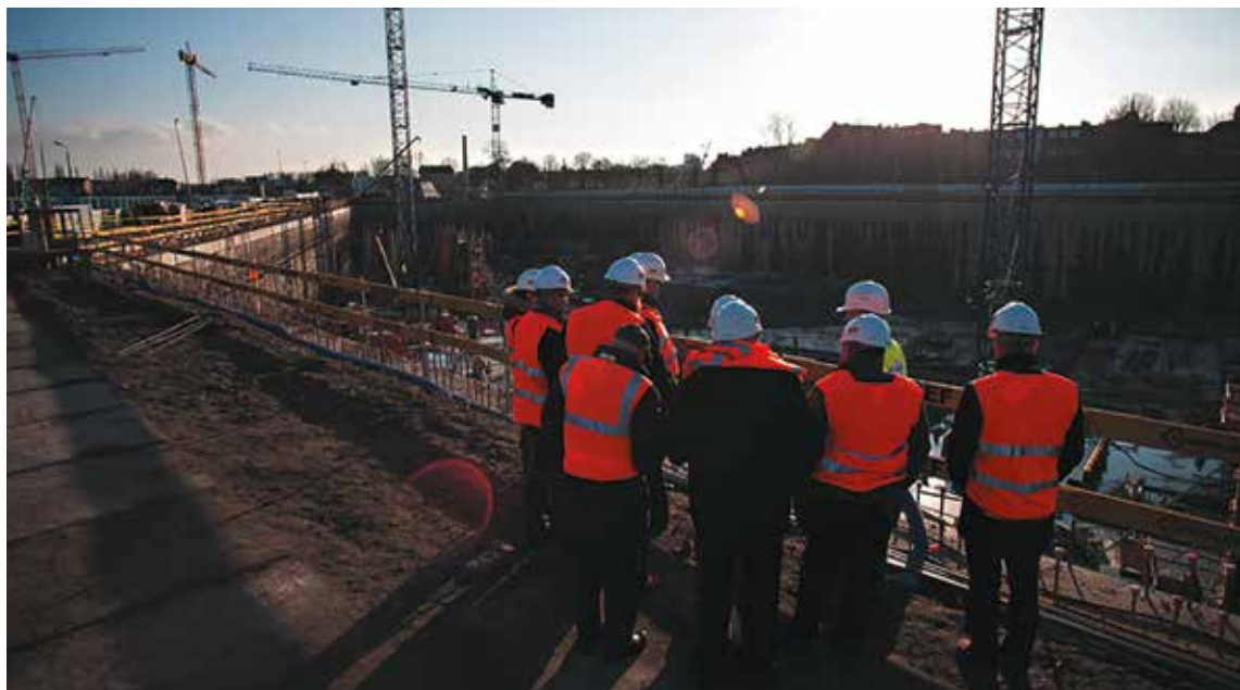
Board of Trustees of the Museum of the Second World War visiting the construction site. 17 December 2014. Photo: Roman Jocher.
