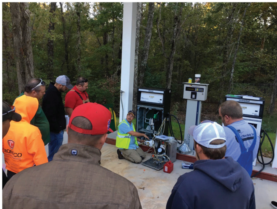
Dale Utke with Purpora Engineering instructing students for line tightness testing technician certification
