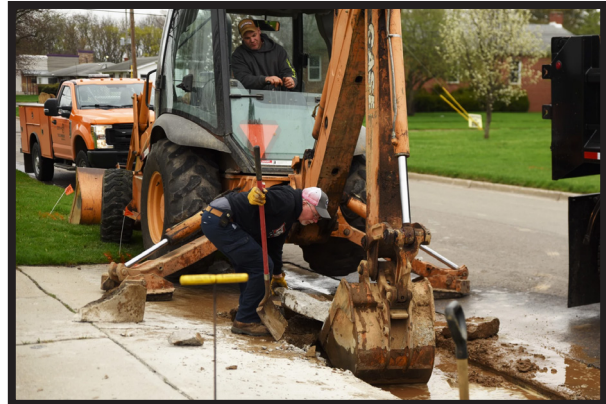
In partnership with the Great Lakes News Collaborative, Michigan Radio published a series of stories titled "Water's True Cost." Here, a City of Tecumseh crew excavates to get to a broken water main (Lester Graham).
