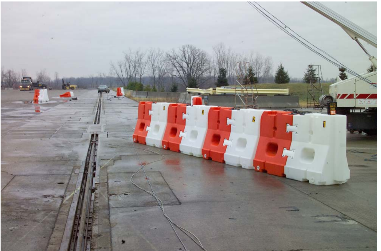
Figure A-41 Post-Test Channelizing Barricade Impact Side Downstream Overall - View 1
