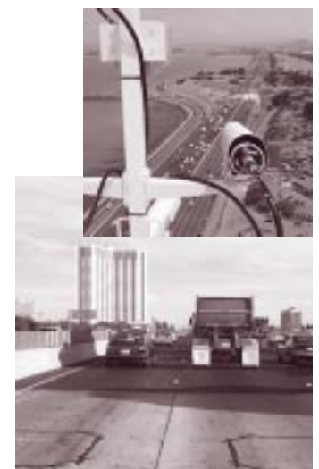
Cameras Placed on top of the Pacific Park Plaza Building
