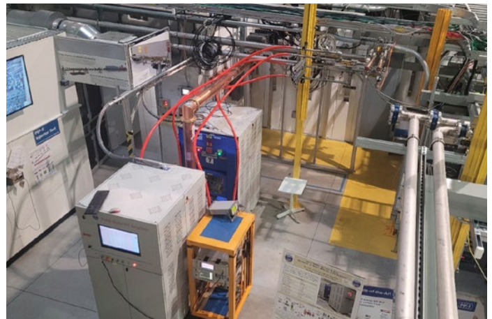
40 kW, 650 MHz Solid State Amplifier (two cabinets) in the CMTF building. Credit: Victor Grzelak
