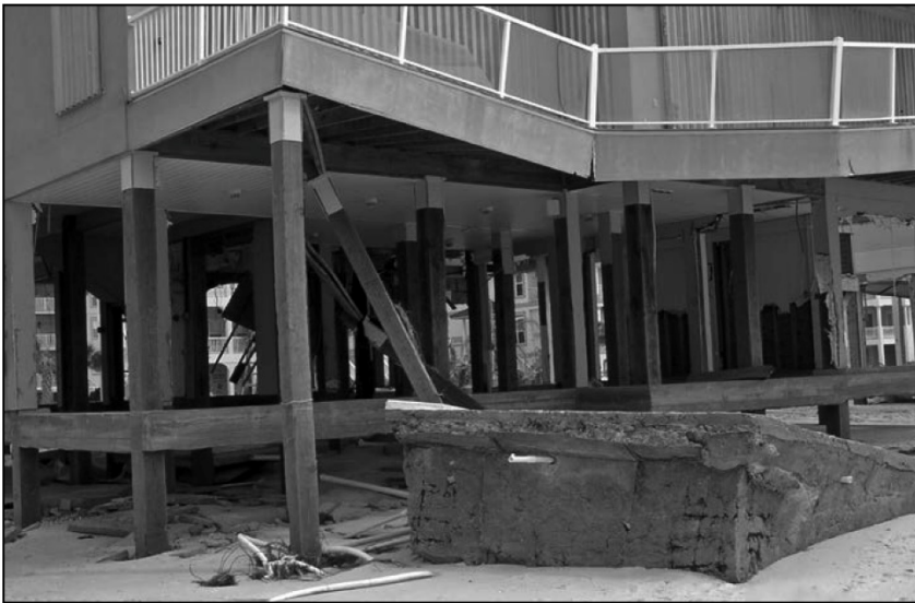
Figure 28: Failure of two piles supporting an elevated deck that was likely caused by movement of a spa
