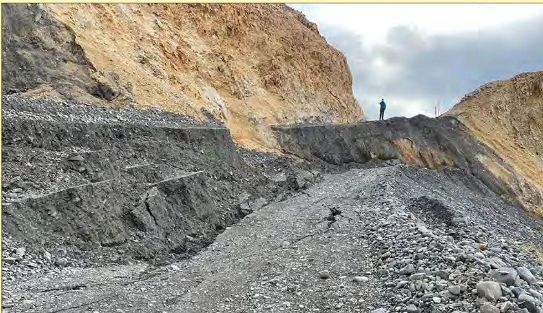
Slow-moving landslides can have equally damaging effects on infrastructure as those that happen quickly. In August 2021, National Park Service officials in Denali National Park, Alaska, were forced to close the only major road in and out of the park for the remainder of the summer season because of downslope movement of the roadbed. In the two weeks following the closure, the road dropped approximately 14 vertical feet (National Park Service, 2021). Photograph by the National Park Service.
