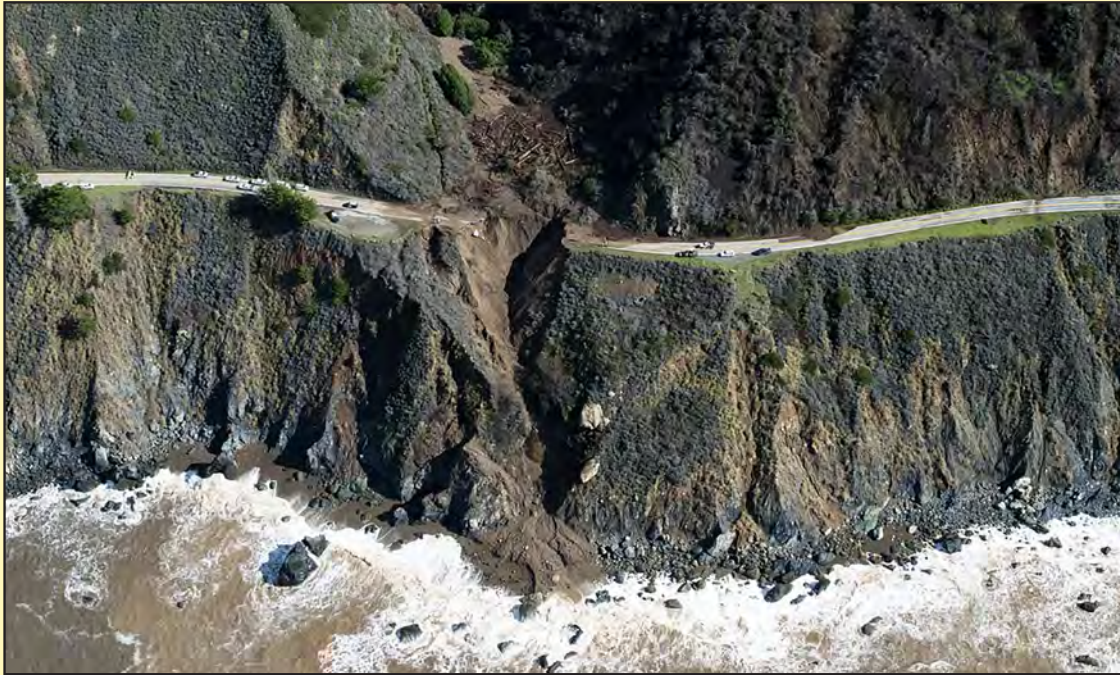
A storm that hit California's coast between January 26 and January 28, 2021, destroyed a portion of Highway 1 near Big Sur. A U.S. Geological Survey reconnaissance flight captured this photograph above the Rat Creek drainage showing the debris flow that damaged the highway. Photograph by the U.S. Geological Survey.
