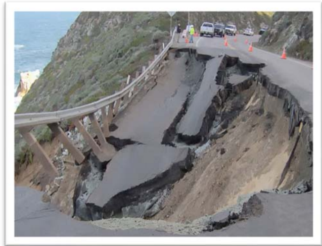
Landslides caused by heavy rain weakened the foundation of Pfeiffer Canyon Bridge, causing it to crack and start sliding down the hillside in February 2017 (Credit: California Department of Transportation)
