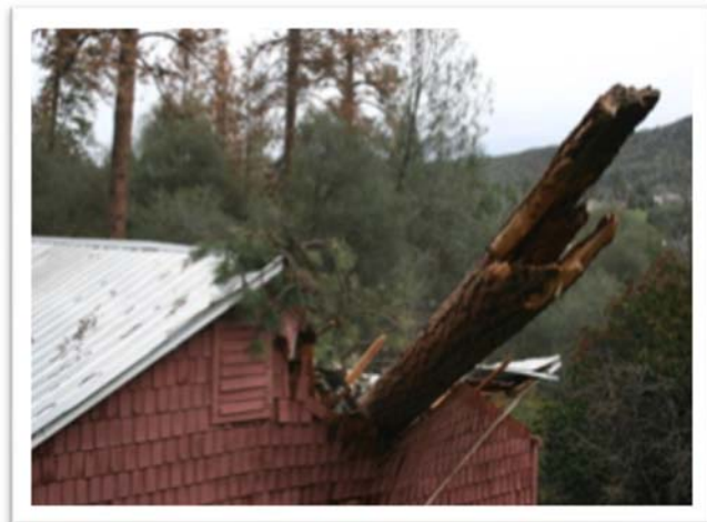
Home impacted by a distressed tree post-wildfire (Credit: CAL FIRE)
