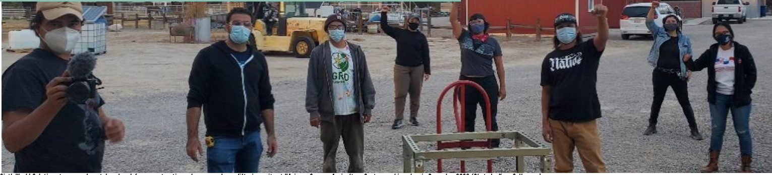
Sixth World Solutions team members take a break from constructing solar-powered nanofiltration units at UArizona Campus Agriculture Center machine shop in December 2020 (Photo by Kern Collymore)
