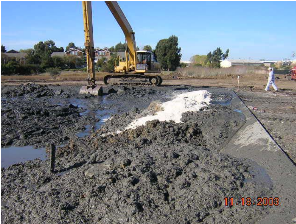
M1A SEDIMENT MIXING IN CONCRETE PAD
