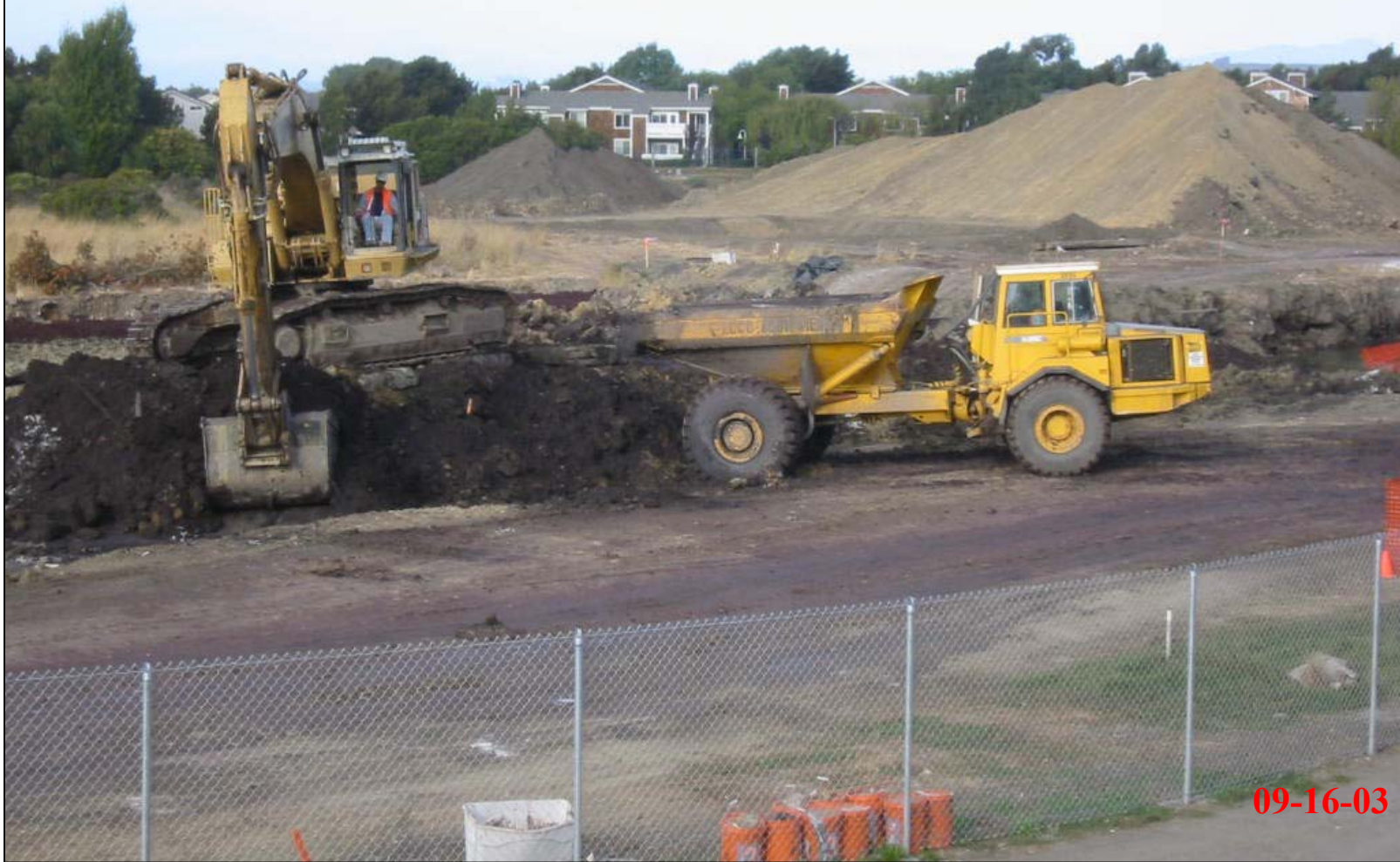
Contaminated soil is excavated using excavators and transported using 25- and 35-ton capacity haul trucks.
