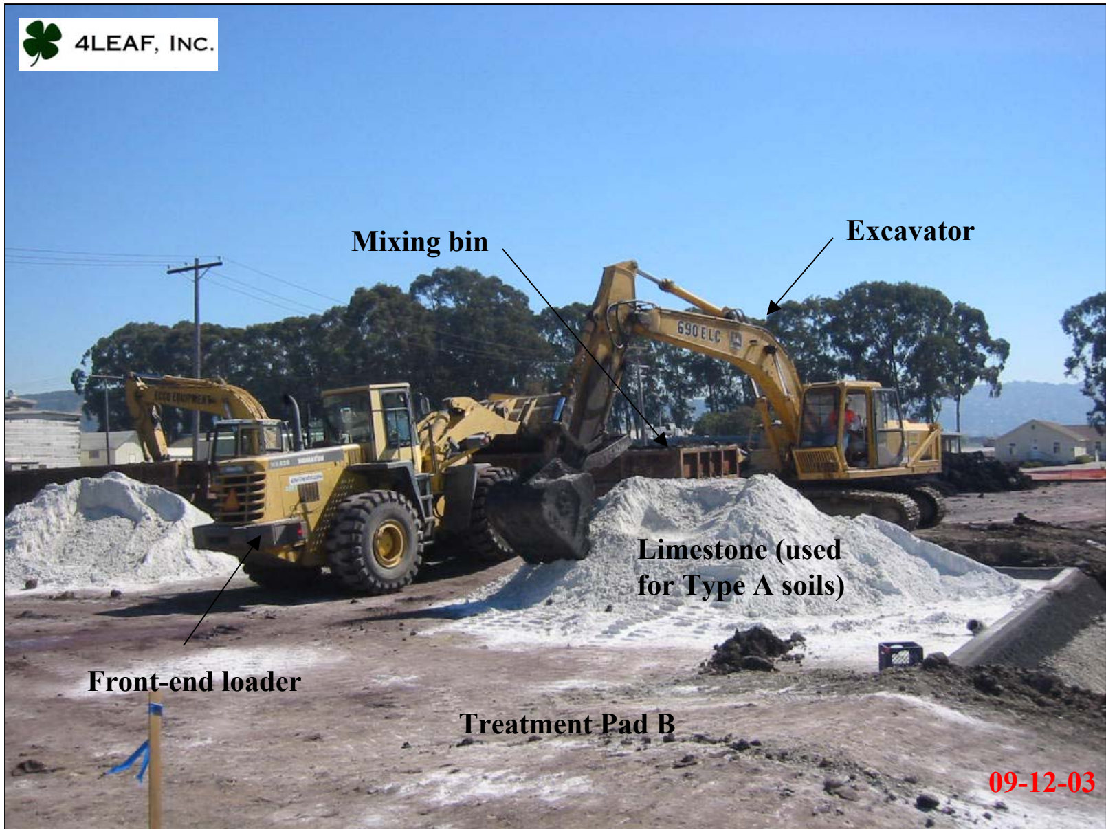
The front-end loader places a measured amount of contaminated soil and reagent into mixing bin.
