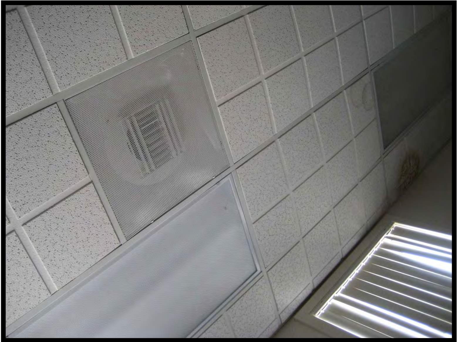
163-02, view of ceiling, vent directly above sample location.
