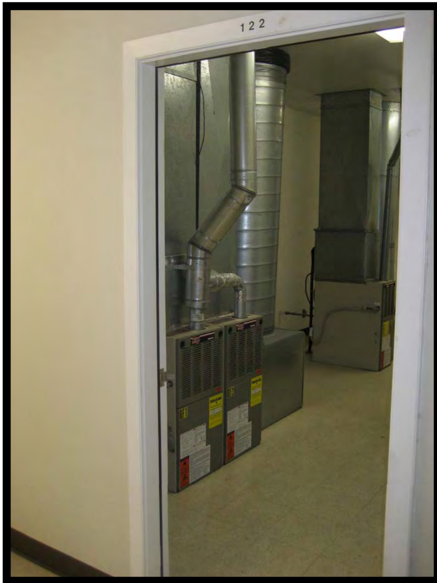
163-01, mechanical room, located directly across hall from sampling location
