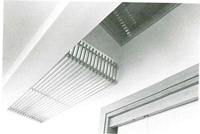
Alcove reading light. Fluorescent strip lamp covered by fir slats. The light is integrated with a skylight to allow for both natural and artificial lighting of the area.
