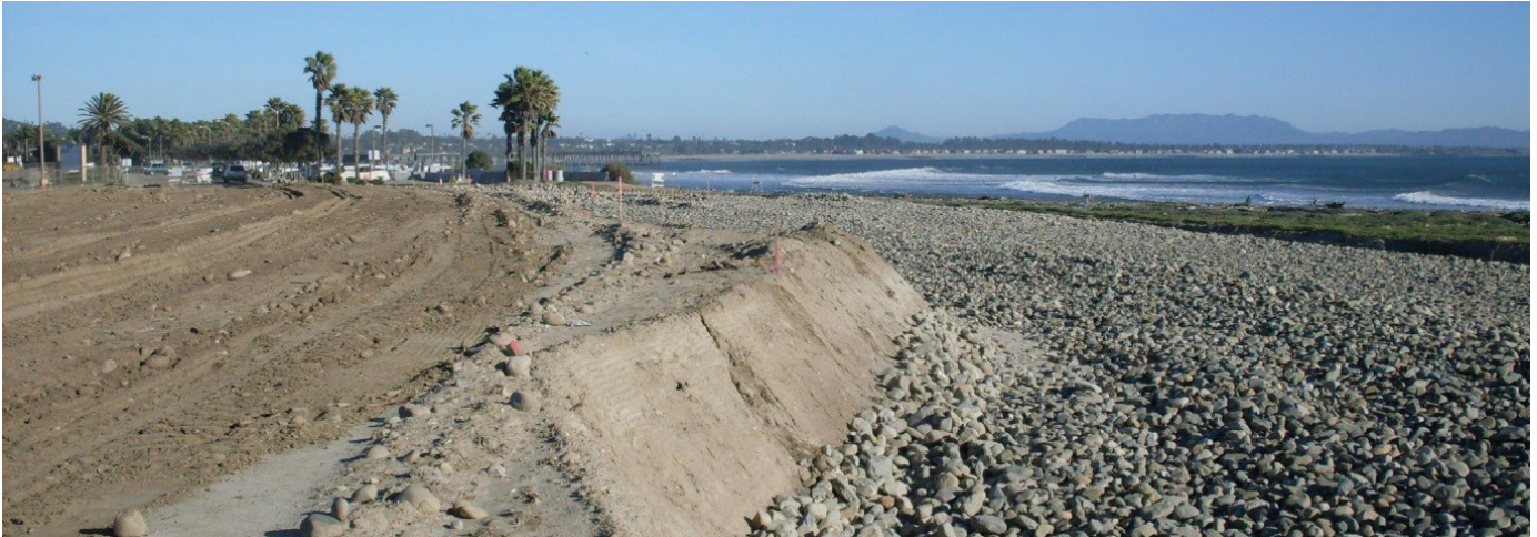
▲ Figure 13: After the eroded parking lot and bike path were excavated, cobble was imported and covered with sand to restore the cobble beach. 2011. Photo credit: City of Ventura.
