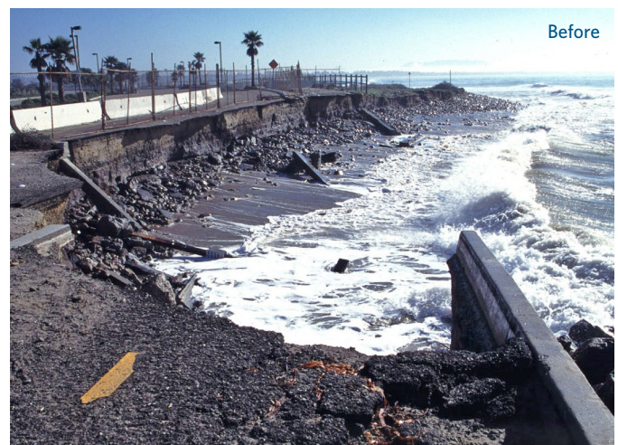
▲ Figure 9: Project site before landward realignment of built infrastructure and restoration of the dunes and beach. The bike path and parking lot were built on fill in 1989 and eroded within 2 years. Photo credit: Paul Jenkin.
