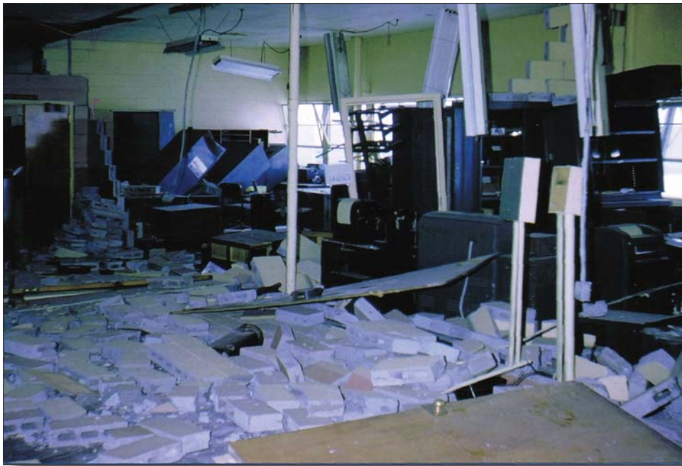
Shaking damage in the U.S. Weather Bureau office at Anchorage International Airport during the 1964 earthquake. Note the failure of unreinforced concrete masonry unit (CMU) walls and extensive nonstructural damage. Photo by A.L. Comiskey.
