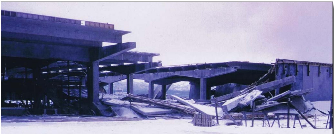
Alaska Sales and Service automobile dealership under construction in Anchorage. The precast concrete wall, column, and roof structural system was toppled by ground shaking during the 1964 earthquake. Photo by A.L. Comiskey.
