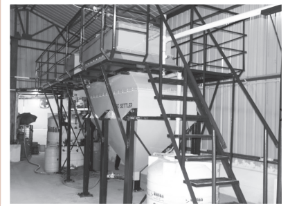
ECAR pilot plant, Dhapdhapi High School, Kolkata
