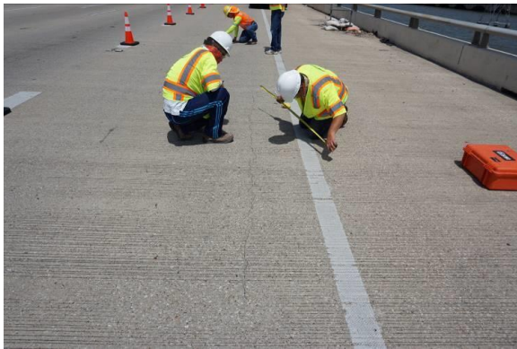
Longitudinal crack on Bridge Deck #9
