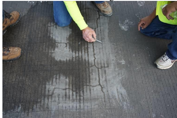
Map crack pattern on Bridge Deck #9
