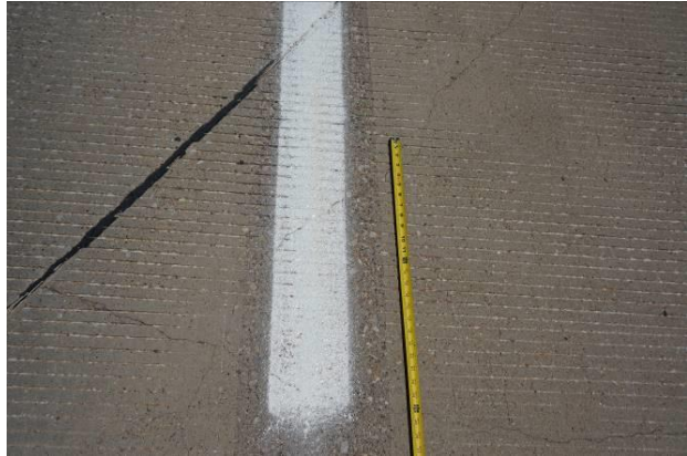
Transverse Crack Propagation on Bridge Deck #7
