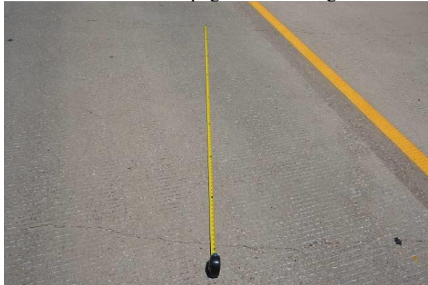
Diagonal Crack Propagation Bridge Deck #7
