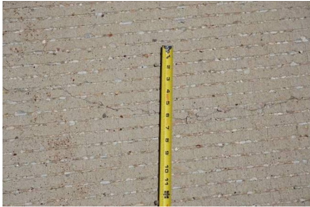
Transverse Cracks on Bridge Deck #6
