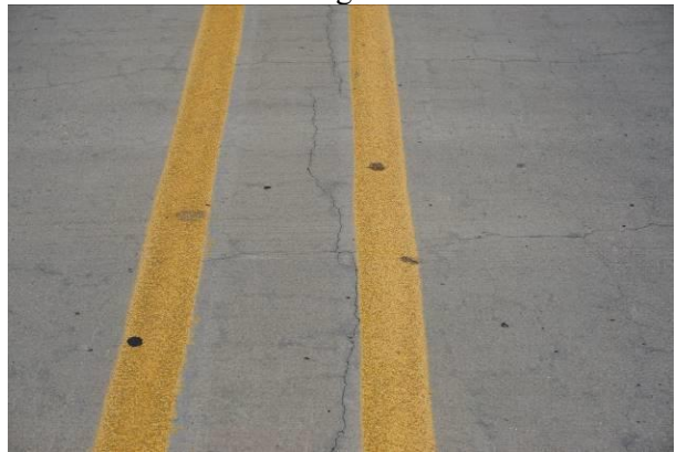
Longitudinal crack propagation for full length along centerline of the Bridge Deck #5
