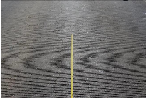
Longitudinal Crack on Bridge Deck #6
