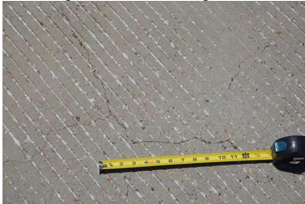
Map Crack Pattern on Bridge Deck #7
