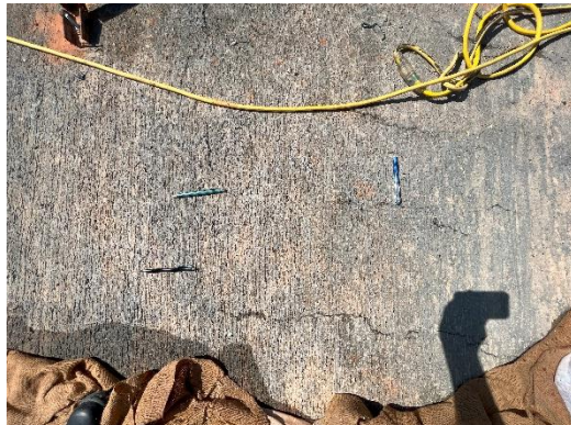
Isolated cracks on deck—FM 2277
