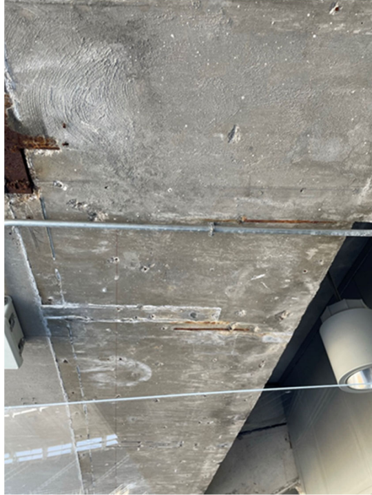
Figure S-4: Rusted Metal in Support Frame Location: Middle Concourse
