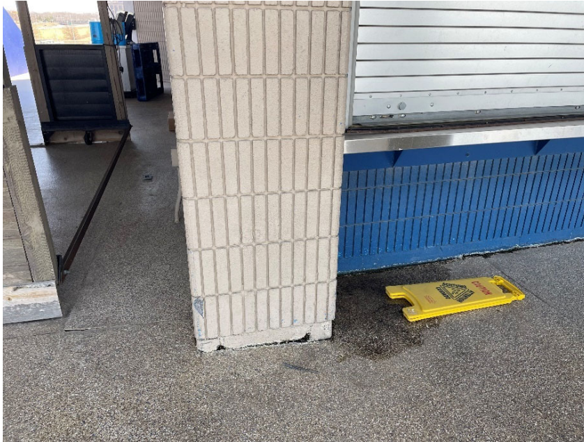
Figure C-4.1: Concession Stand, Holding Water Location: Upper Concourse Concessions Stand
