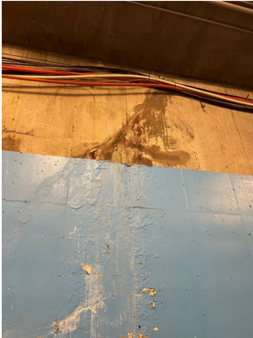
Figure S-1: Water Damage
