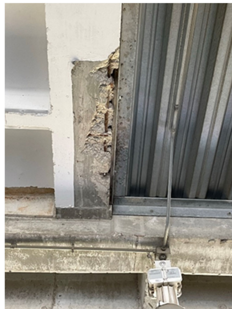
Figure S-3.2: Support Frame Deterioration Location: Middle Concourse
