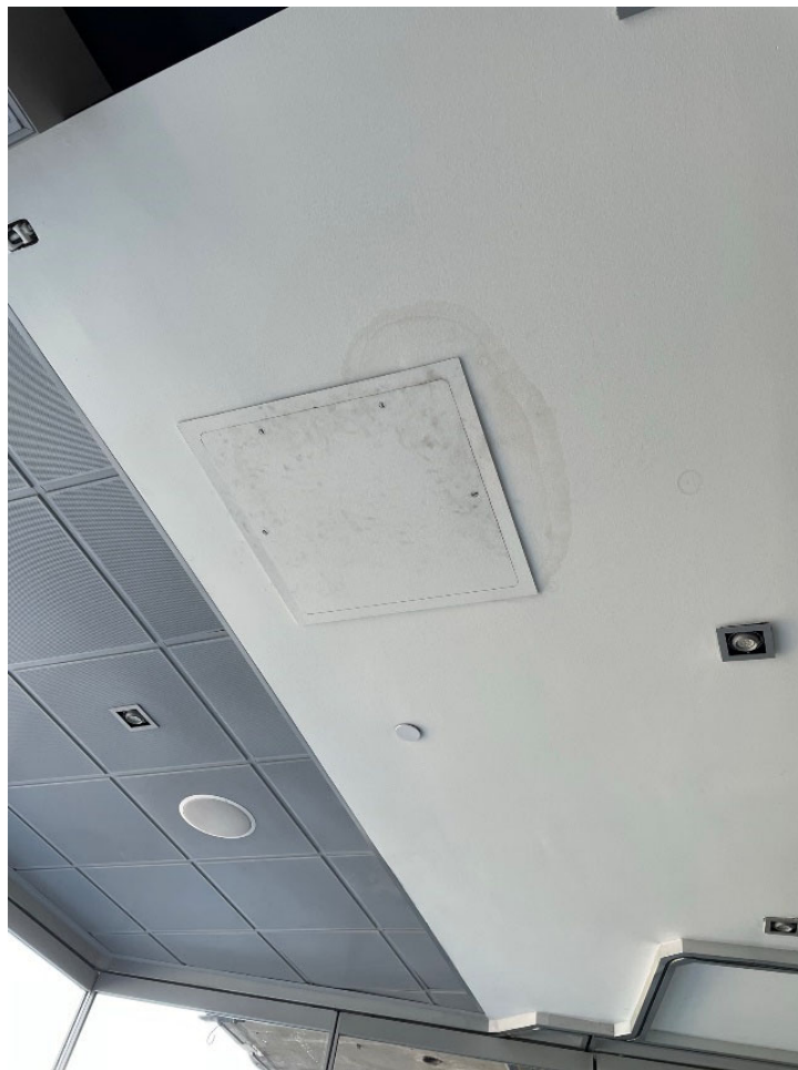
Figure AI-3: Water Damage Location: Diamond Club
