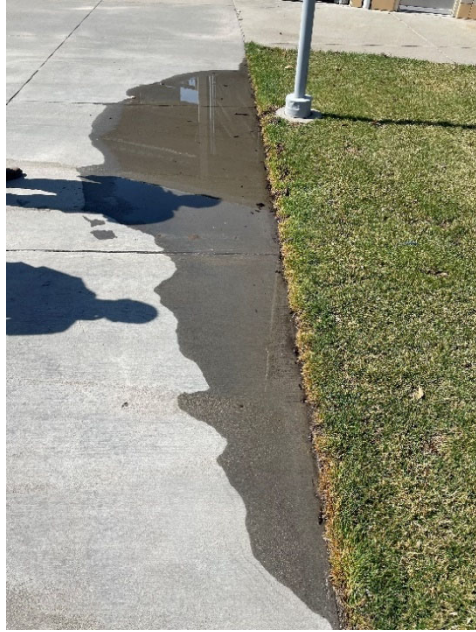
Figure C-2: Water Ponding Location: Near Gate A
