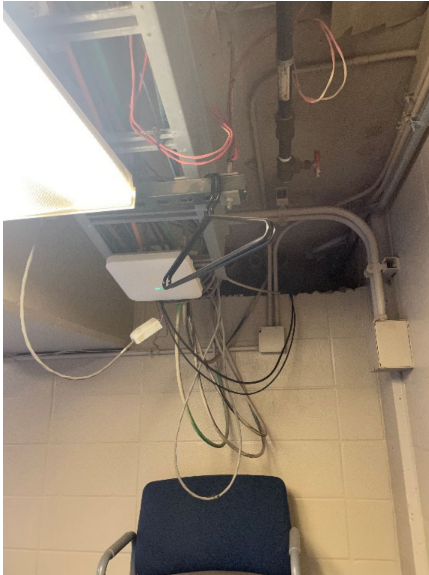
Figure C-11: Cable Management Needed Location: Tunnel by Dugout
