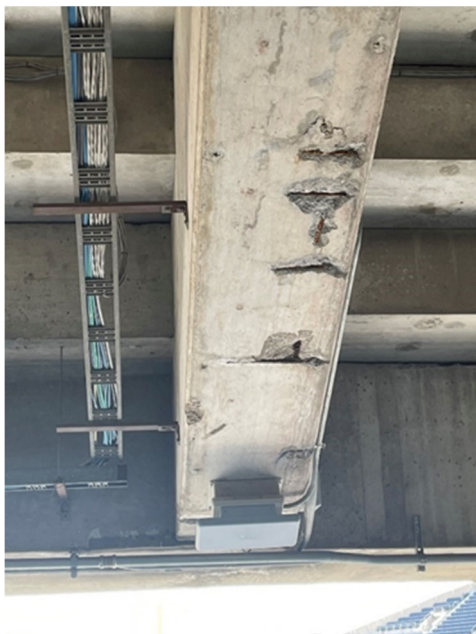
Figure S-3.1: Support Frame Deterioration Location: Looking Out From H&R Block Private Suite
