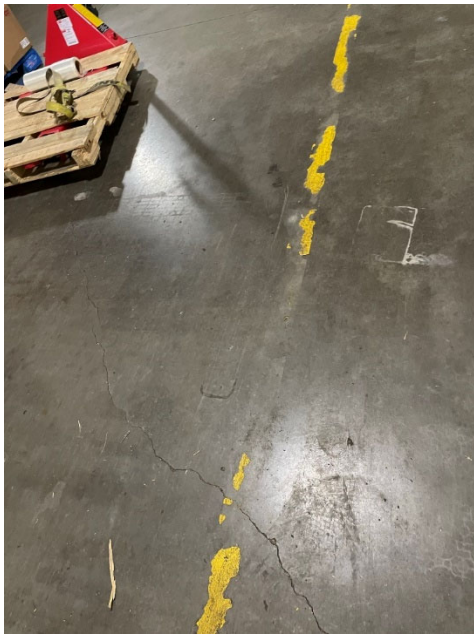
Figure AI-1: Caution Strip Location: Back of House Food Storage
