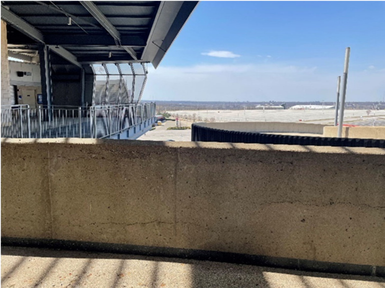
Figure S-7: Wall with Horizontal Cracks Location: Upper Concourse Near Helix Ramp
