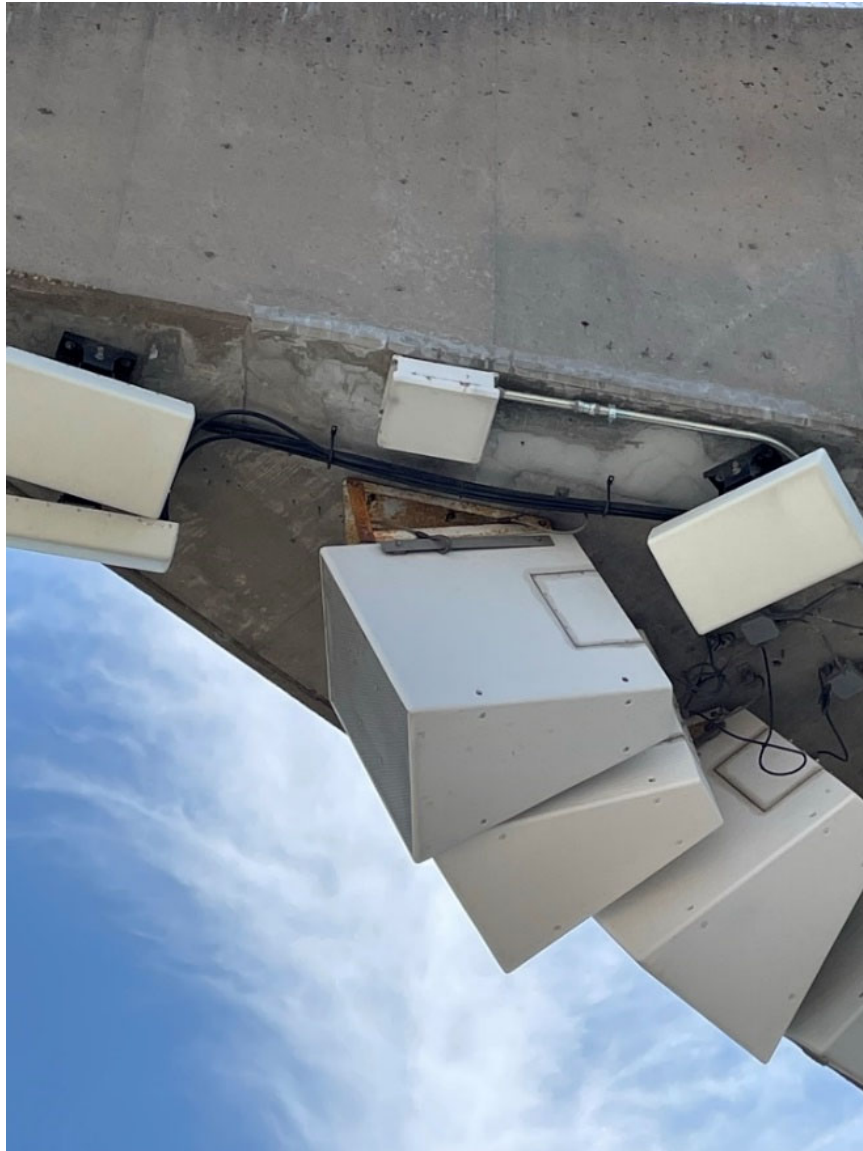
Figure AME-1: Surface Rust on Platform Support Brackets Location: Section 201 Looking Up
