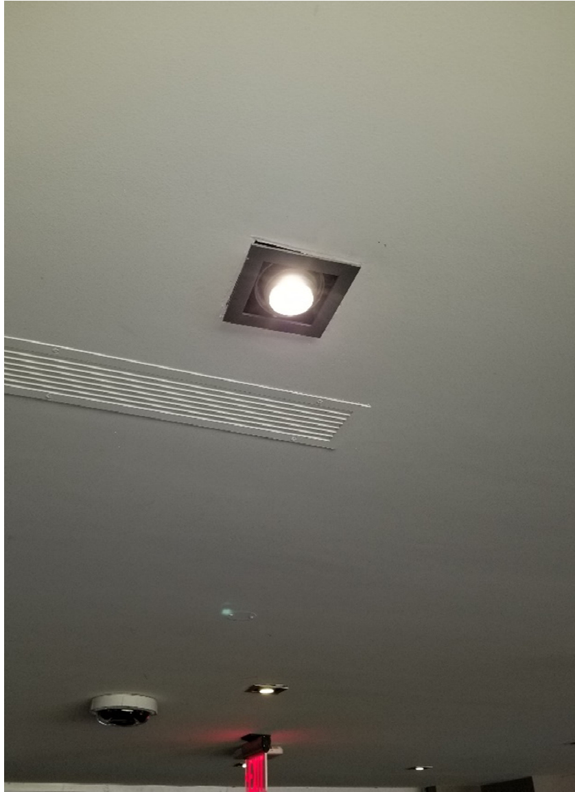
Figure E-2: Ceiling Mounted Fixture Location: Kauffman-Arrowhead UG Tunnel
