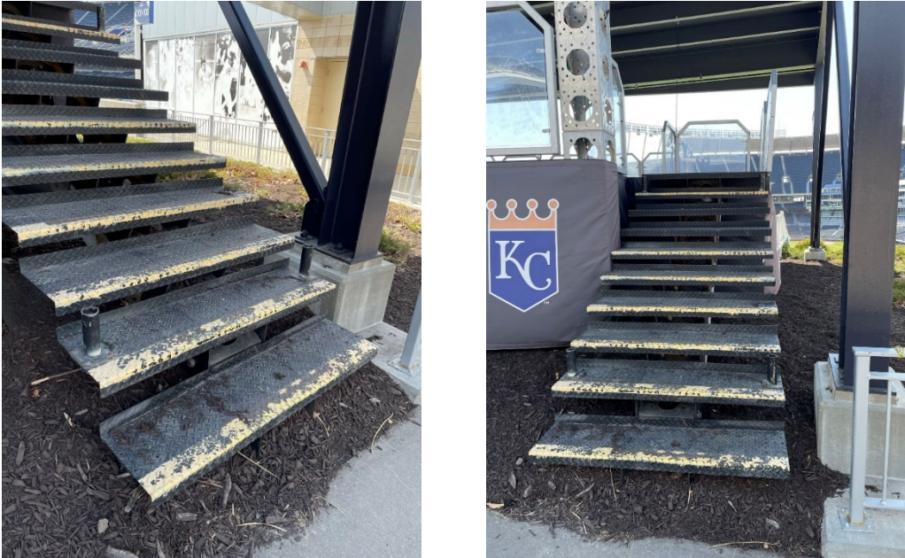
Figure S-8: Missing Handrail Location: Miller Lite Fountain Bar Deck
