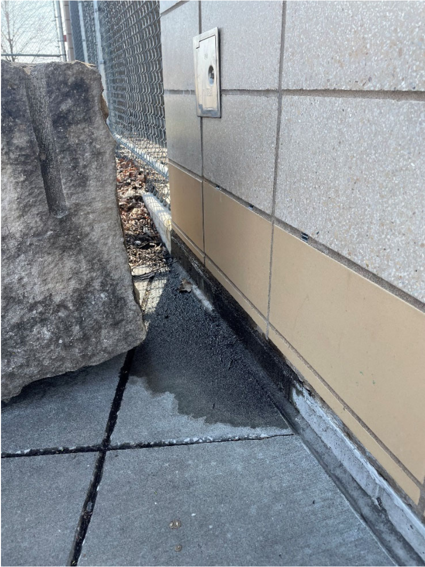
Figure AME-3: Deteriorating Sealant Location: Janitor's Closet J251 – Outfield Experience
