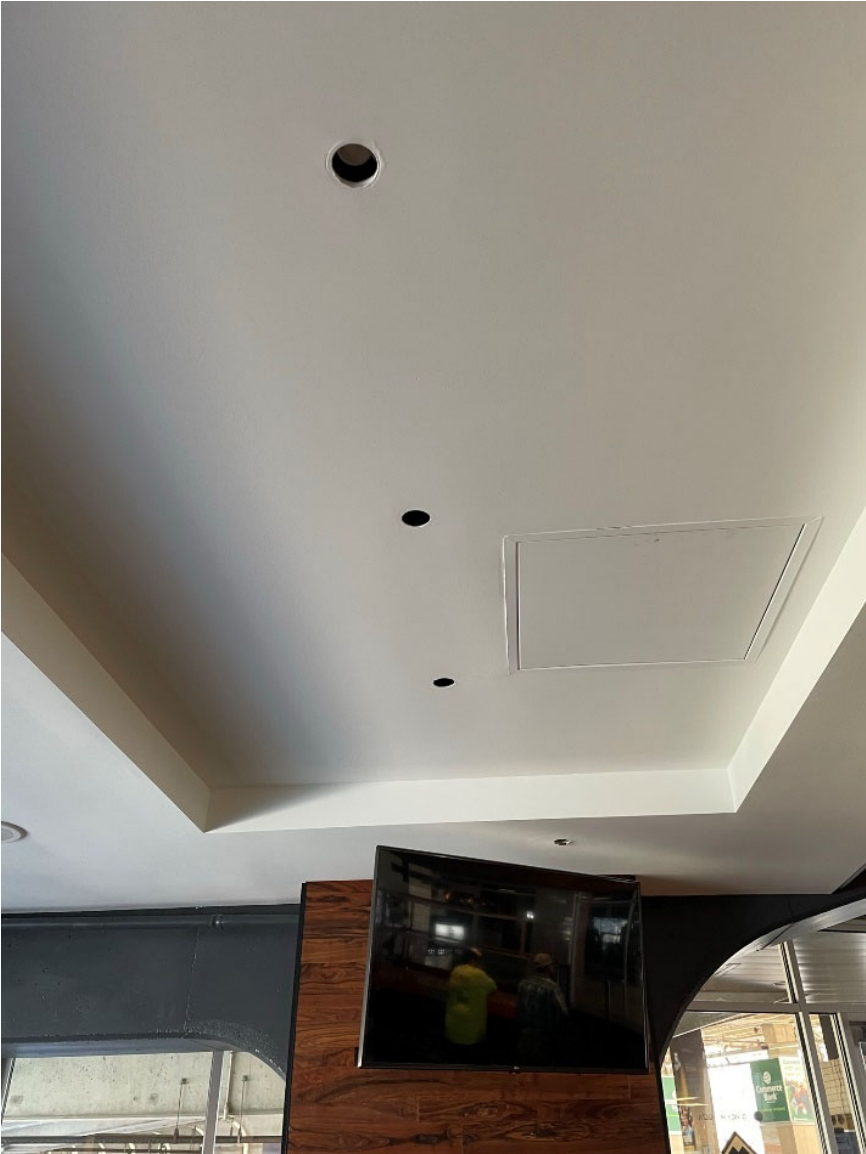
Figure AI-4: Missing Light Fixtures Location: Diamond Club
