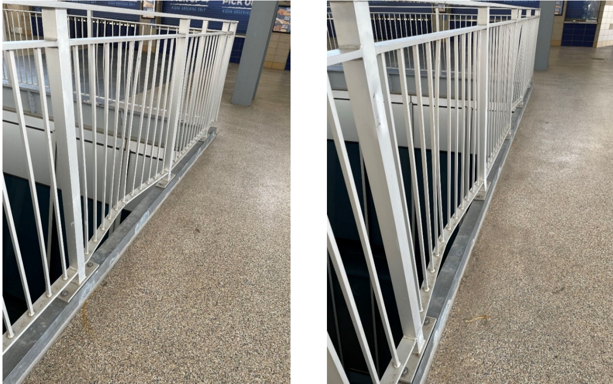
Figure AME-2: Damaged / Bent Guardrail Location: Section 417
