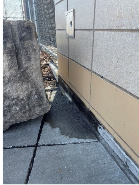
Figure C-3.1: Water Seepage Location: Janitor's Closet (J251)
