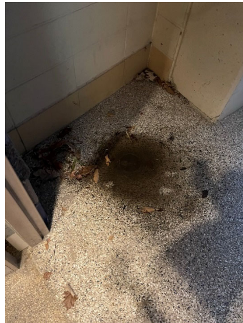
Figure C-5: Water Ponding Location: Women's Restroom, Around Section 216
