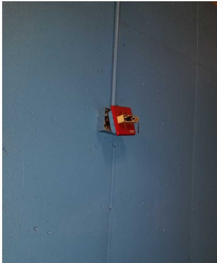
Figure E-1: Fire Alarm Strobe Location: Kauffman-Arrowhead UG Tunnel
