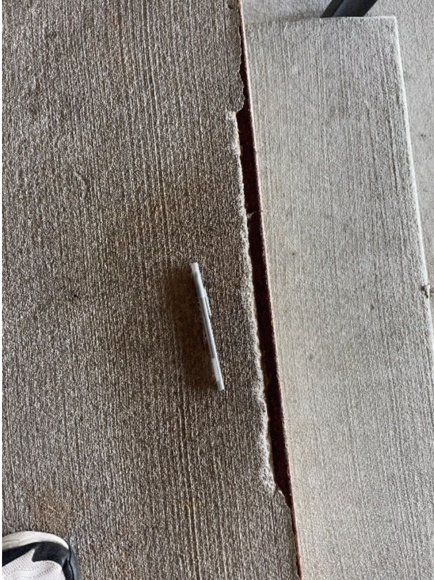
Figure C-8: Eroded Step Edge Location: H&R Block Private Suite Stairs
