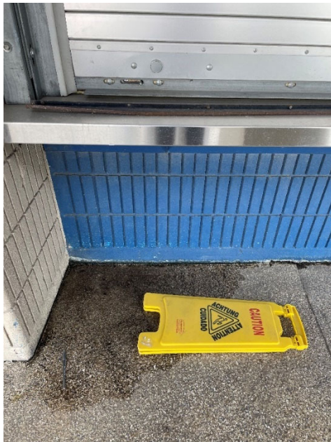
Figure C-4.2: Concession Stand, Holding Water Location: Upper Concourse Concessions Stand
