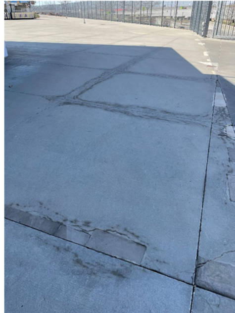
Figure C-1.2: Concrete Cracking Location: Unknown
