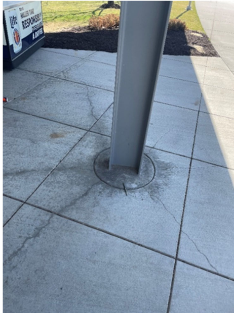
Figure C-1.1: Star Cracking at Column Foundation Location: Outfield Plaza
