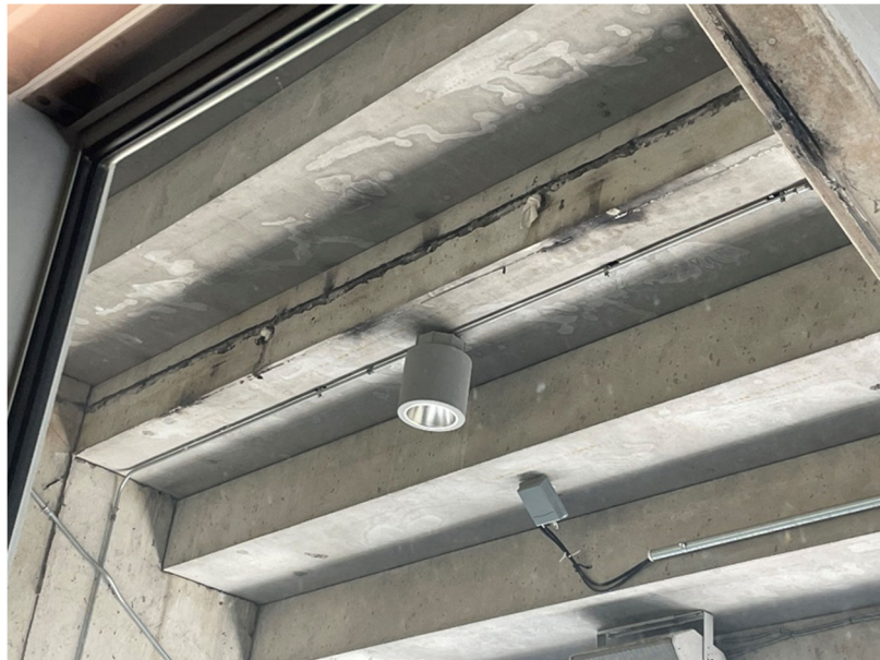
Figure S-5: Support Frame Deterioration Location: Looking Out From H&R Block Private Suite
