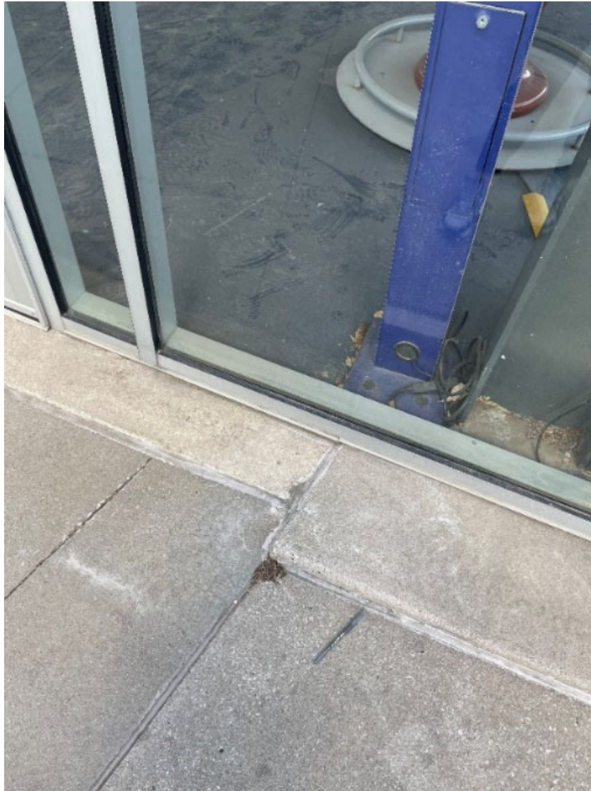
Figure C-7: Tripping Hazard, Uneven Pavement Intersection Location: Adjacent to Miller Lite Fountain Bar
