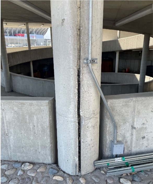
Figure S-6: Support Column Caulk Deterioration Location: Gate D
