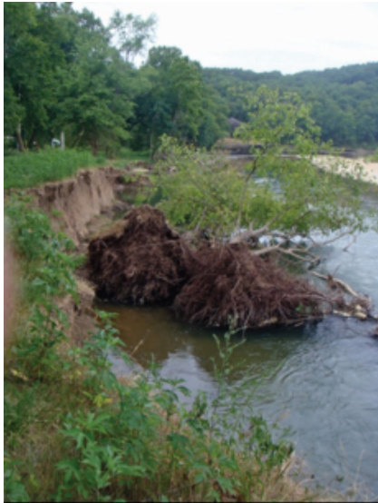
Figure 4. A tree toppling into a river is a sign of a mass bank failure.
