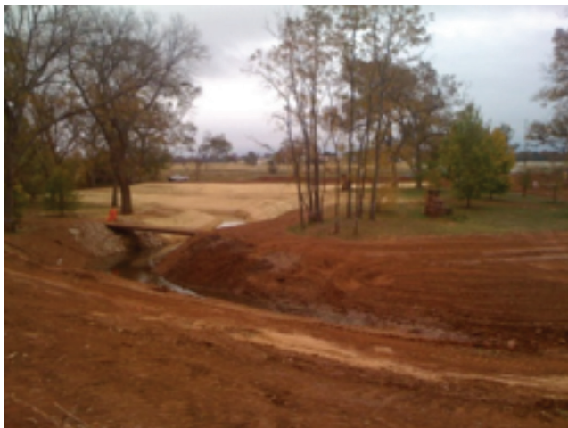
Figure 6. A bank that has been re-sloped. Vegetation will be added once construction is complete.
