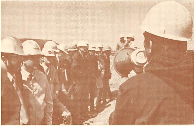
It took 15 million cubic yards of sand to fill and surcharge 300 acres of marshland. . . .
