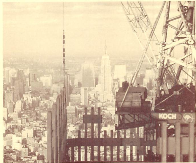
1970 Photograph of steel erection at the 103rd floor of the World Trade Center
