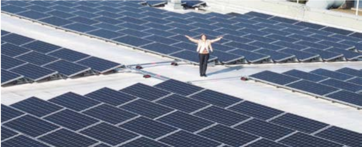
Chief Sustainability & Carbon Solutions Officer Kira Stoll celebrating the rooftop solar array on the Recreational Sports Facility.
