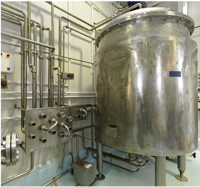
Figure 3. This is an example of a bulk or batch pasteurizer typically used to pasteurize product all at once and/or after being packaged. (Photo courtesy of Markobe from Adobe Stock)
