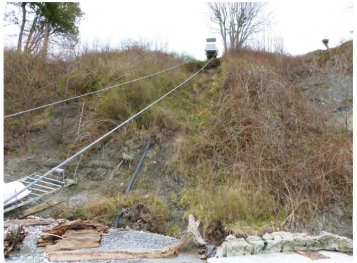
Gabion removal area in 2012 showing both immature vegetation and recent slope failures.
