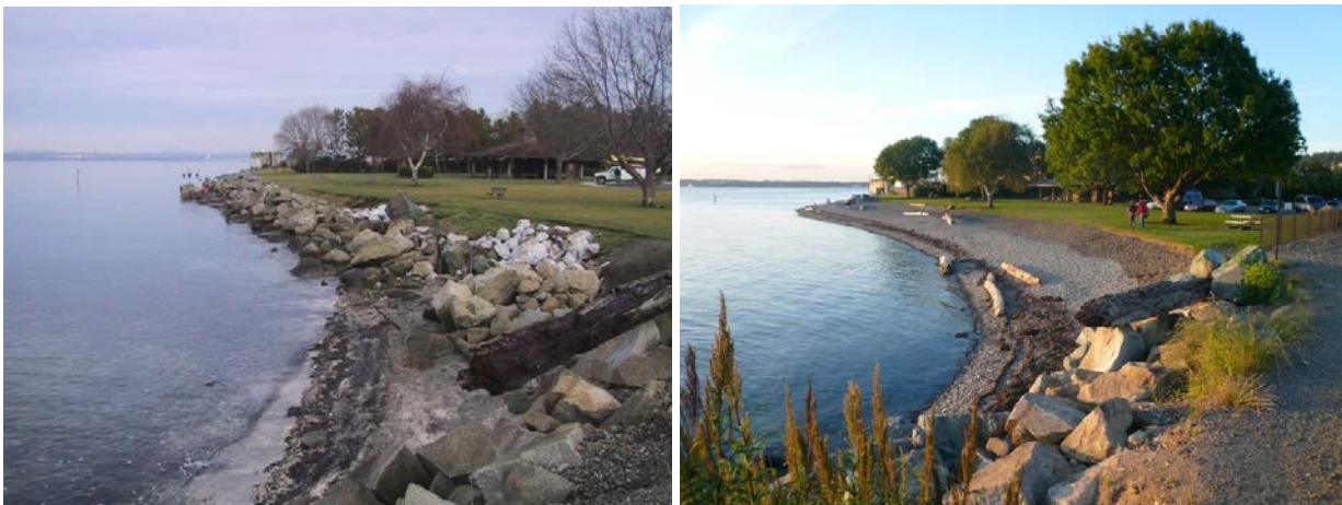
Figure 5-3. Before (left, 2004) and after construction (right, 2007) at Marine Park in Bellingham, Washington. This project is an example of multiple design techniques employed at one site: bulkhead and partial fill removal, with beach nourishment and a rock drift sill to contain sediment (partially visible in far end of beach), and adjacent revetment maintained to protect railway (on right).
