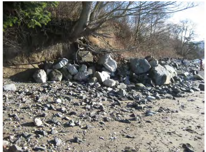
Project site revetment north end in 2012 looking up-drift of the structure end. Note toppled armor rock and quarry spall, which has moved out of the structure.
