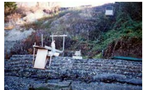
Gabion basket bulkhead in 1999 looking east. Note poorly vegetated bluff face, aerial tram, and lower gabions failing to south (right).
