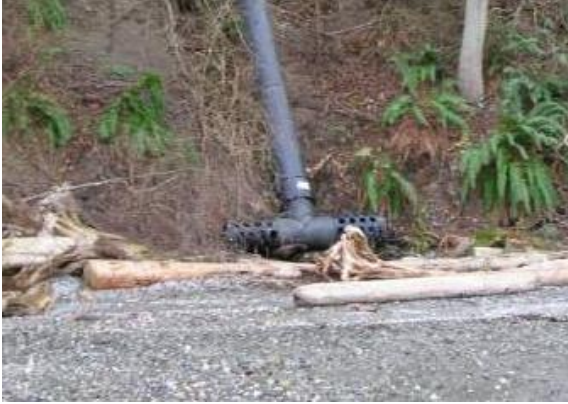
Figure 6-3. Diffuser tee mounted at the toe of the slope, upland of OHW, and behind existing drift logs. No rip rap pad was used.
