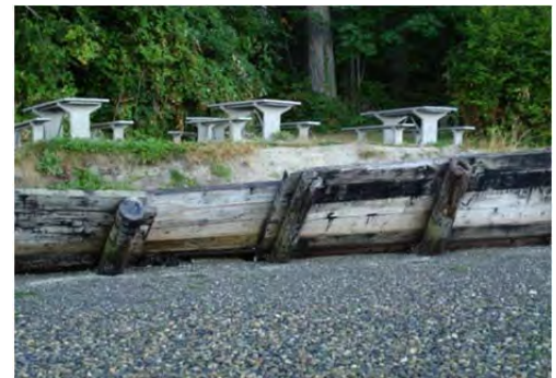
Wooden bulkhead mostly collapsed to expose fill and landslide deposits in 2006. Note waterward lean.
