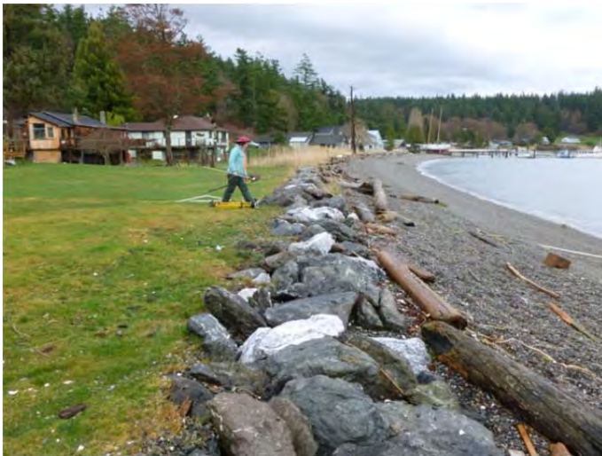
Project site looking down-drift in 2012. Note landward overwash of the revetment, exposed rock and geotextile fabric, and small log zone waterward of structure.
