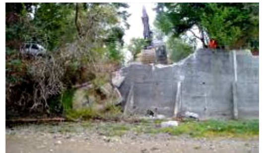
Removal of the concrete bulkhead in progress in 2005 at the western portion of the site.
