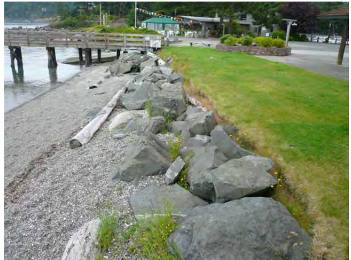
Project site and profile location looking down-drift in 2012. Note rock toppling and lower elevation of eastern portion of revetment.
