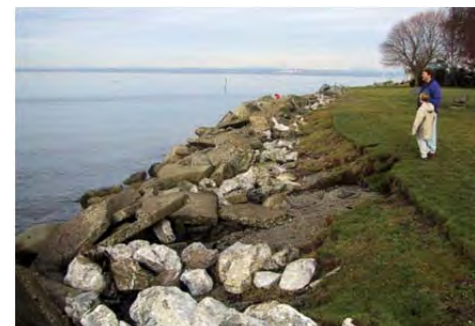
Revetment looking north. Note erosion behind the rock due to wave overtopping. Lighter-colored rock was a more recent addition in response to continued erosion.
