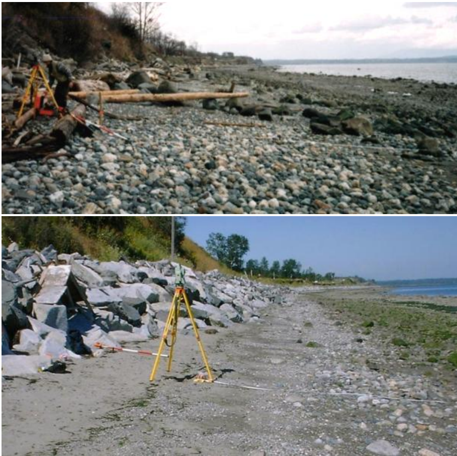
Figure 7.1-14. Lummi Shore Road on Bellingham Bay, Lummi Reservation at the same location in the central reach. Prior to revetment construction (top, 1998) and after (bottom, 2000). After revetment was built beach nourishment was applied for mitigation. However, without continued nourishment, the beach is much coarser in 2014 (J. Johannessen photos).
