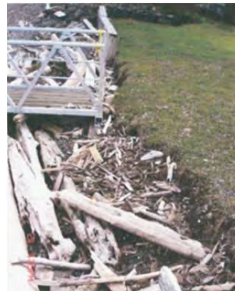
Erosion at dock looking SW, preproject.
