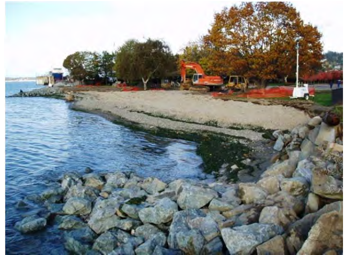
Looking north toward initial grading and placement of gravel between drift sills in early November 2004.
