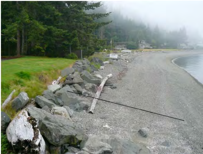
Project site and profile location looking up-drift in 2012. Note toppled rock in foreground and erosion of backshore fill with fewer toppled rocks on beach within the further section of revetment.
