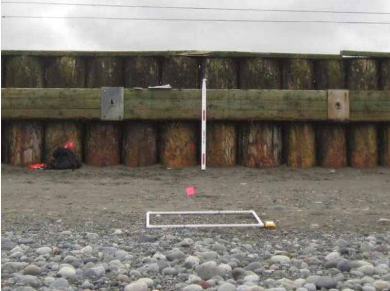
Figure 8-1. Photographic monitoring looking onshore with scalable reference at vertical bulkhead. Photographic monitoring should be done yearly at a minimum in the same location with the same reference. In this case, the same stadia rod or other known length scale should be used. Beach sediment quadrat also in photo for spatial location reference.
