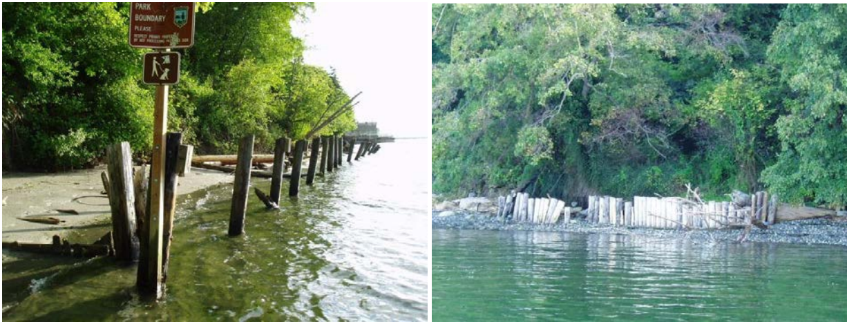
Figure 7.4-2. Degraded bulkheads deteriorating in place.
