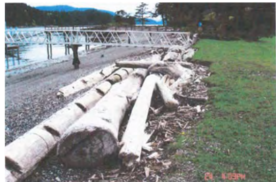
Erosion along shore looking SW, preproject.
