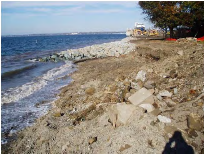
Looking north toward construction of north drift sill and limit of excavation of fill and debris in late October 2004.
