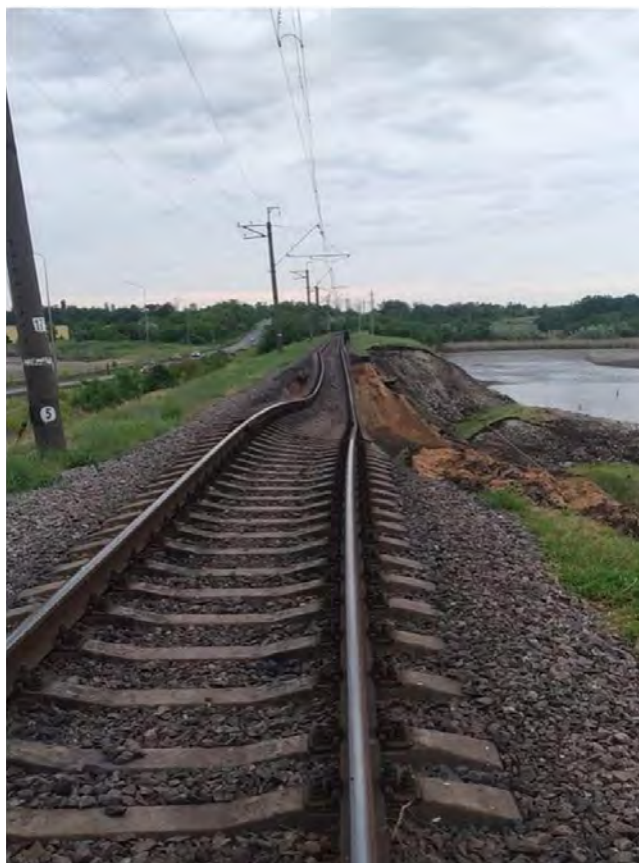
Figure 20. Compressed railroad bed and landslide on the bank of the Kakhovka reservoir after its depletion (near Nikopol) (Source: Yakovlev and Stefanyshina 2023)
